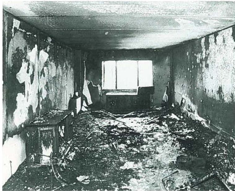
Although the contents of this apartment were destroyed by fire, the concrete walls and ceiling prevented the fire from spreading.
