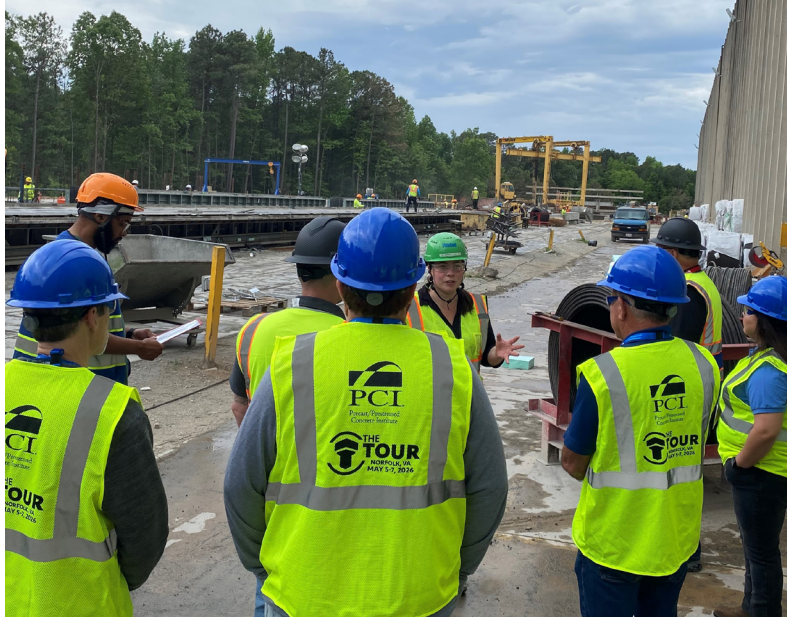
Attendees of the 2026 PCI Productivity Tour learn how Tindall's Petersburg, Va., plant approaches the concrete placement process in their outside production areas. Courtesy of PCI.
