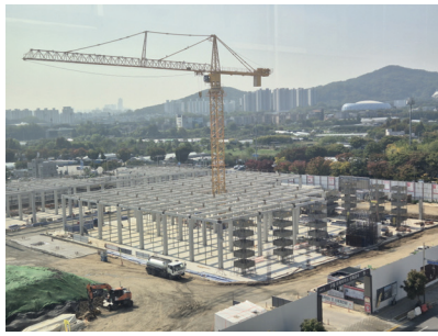
Precast concrete in large warehouse
