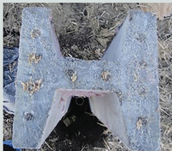
Figure 6.2. Ultra-high-performance prestressed concrete pile end after driving.
