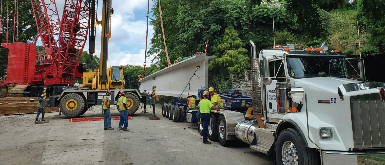
Pennstress delivers a 105-ton (95-tonne) super-load prestressed concrete beam to the Fern Hollow Bridge construction site in Pittsburgh, Pa. Courtesy of Pennstress.
