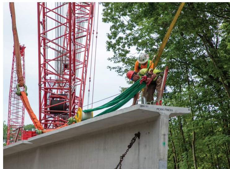
Crews use a small rough terrain crane to position the rigging in preparation for attaching it to the lifting loops embedded in the beam for the new Fern Hollow Bridge. Courtesy of Swank Co.
