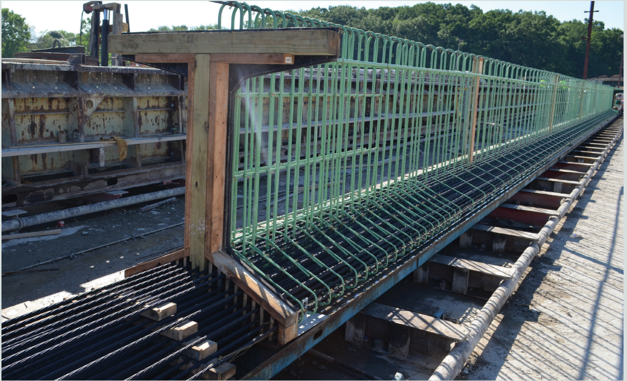
Figure 21. Completing the reinforcement cages of a carbon-fiber-composite-cable prestressed concrete beam for the Brush Street Bridge over Interstate 94 in Detroit, Mich.
