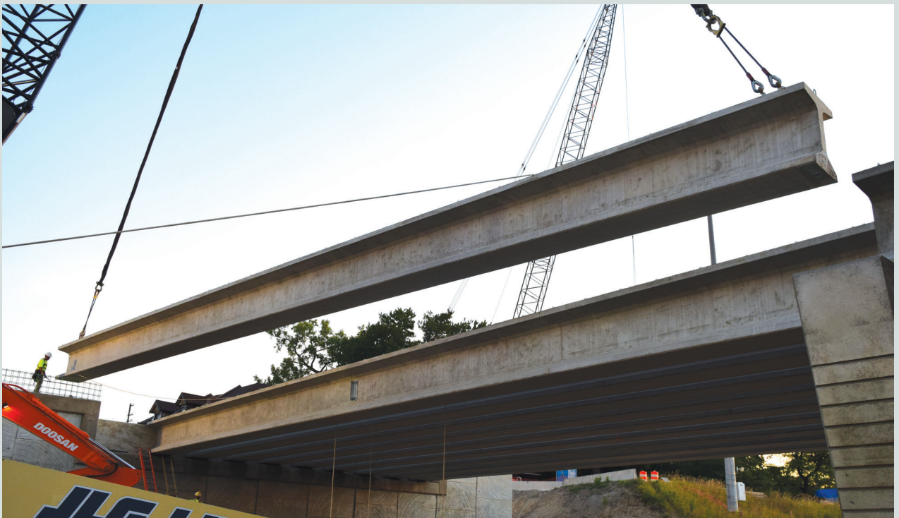
Figure 22. Placing the beams over the supports in Brush Street Bridge over Interstate 94.
