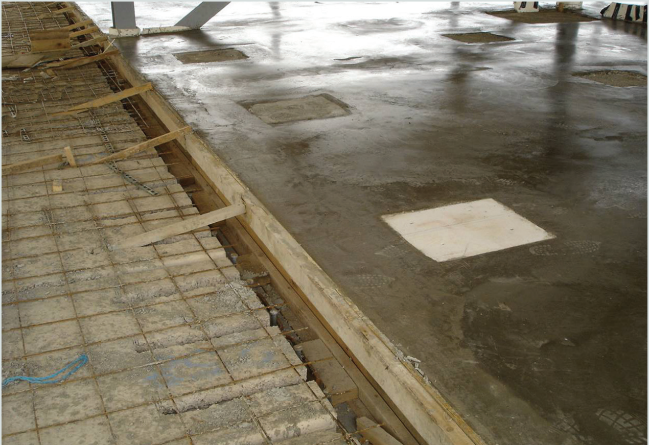
Figure 2 Hollow-core floor slabs (left) prepared with mesh for casting of the structural topping (right). The hollow-core unit should be dampened, without ponding, with water prior to casting the topping. The steel mesh should be lapped with reinforcing bars that are continuous through the construction joint.
