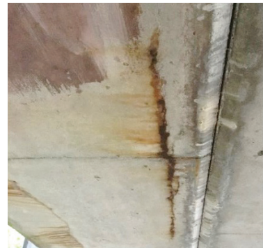
Rust-stained longitudinal crack on north side of beam 1
