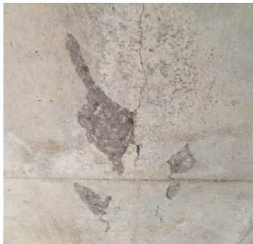
Longitudinal cracking and minor concrete spalling in west end of beam 7
