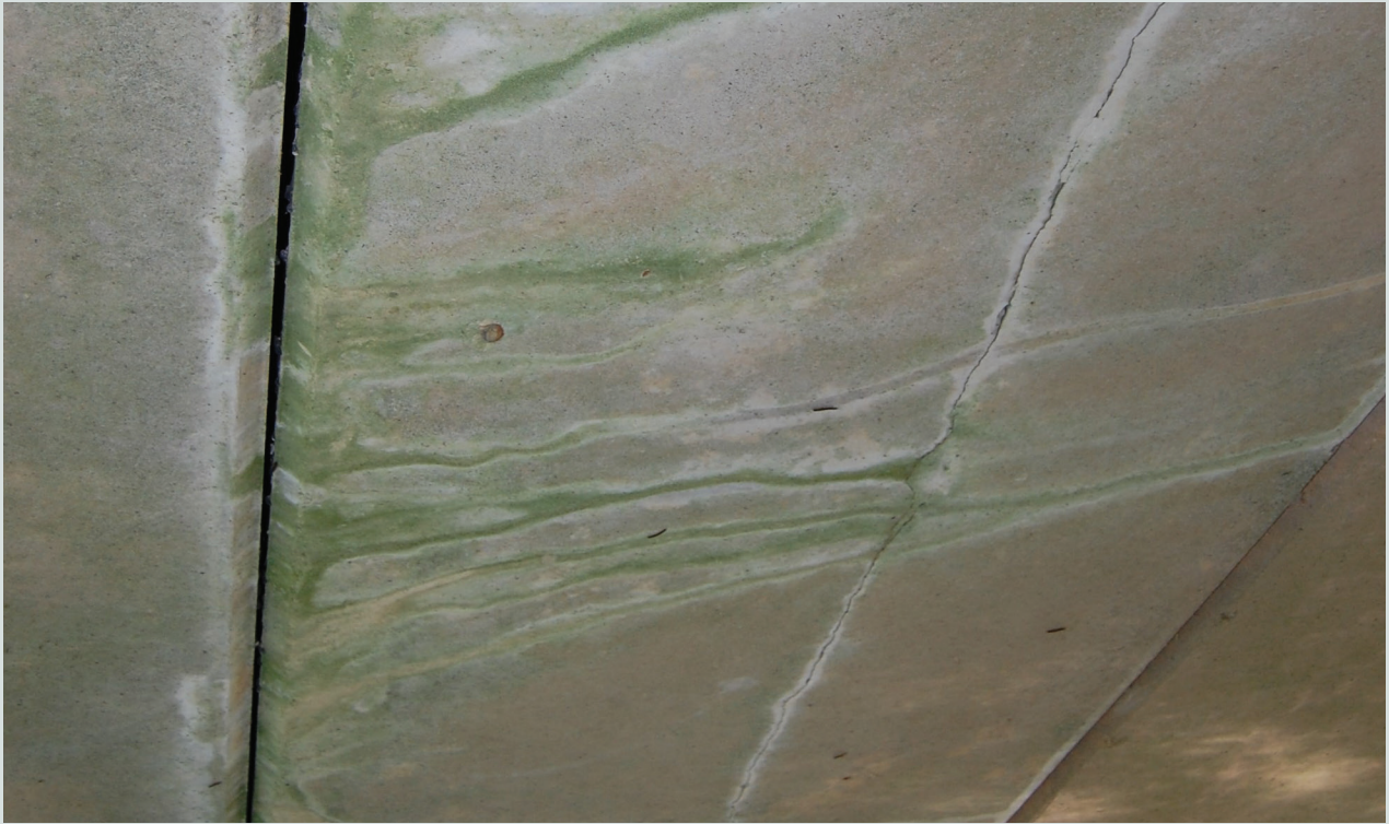
Figure 1. Leaking joint of an adjacent box-beam bridge.
