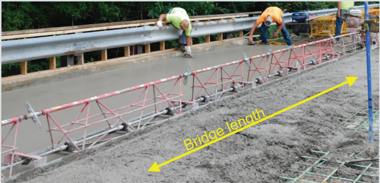
Figure 9. Use of mechanical screed and tapered formwork to construct bridge cross slope.
