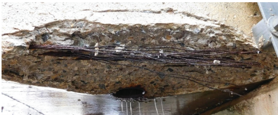
Three exposed strands at east support of beam 1
