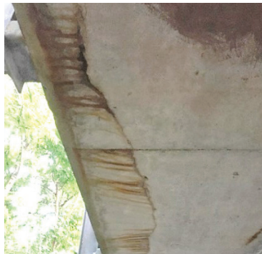
Rust-stained longitudinal crack on south side of beam 1
