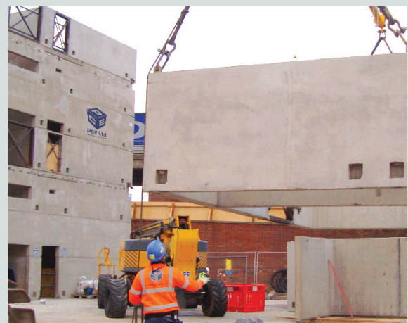
Figure 10. Blockouts for through bolt connections are seen along module edges. Courtesy of PCE Ltd.
