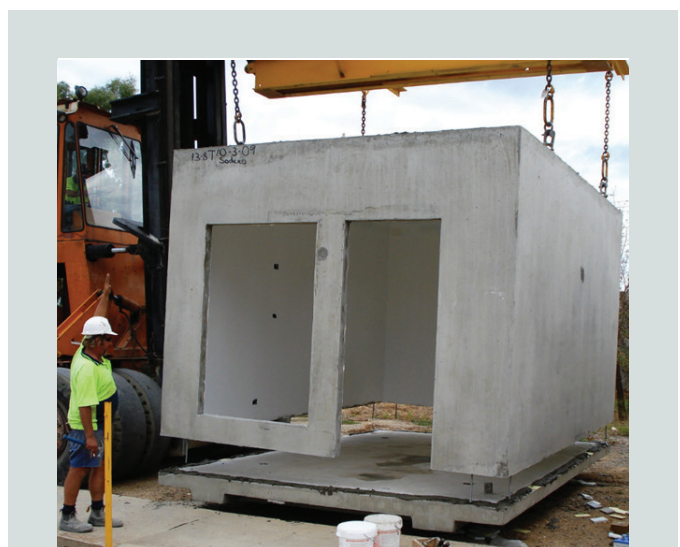
Figure 8. Simple gravity dowel connections on grout pad. Courtesy of Zebra Constructors, Australia.
