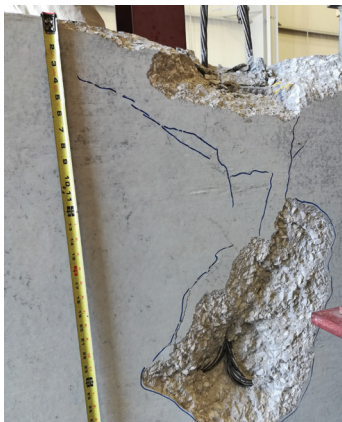
Close-up of side face blowout in B30-1
