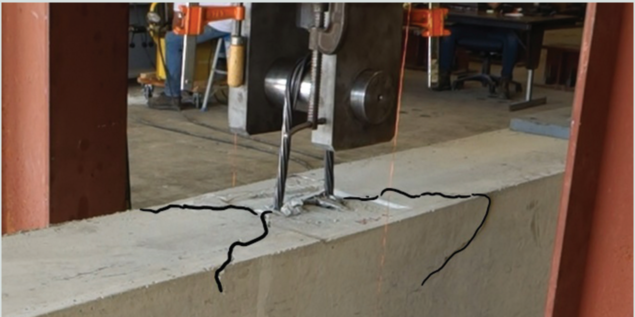
Figure 8. Initial cracking for B24-2. Cracks have been emphasized (traced) for clarity. Note: B24-2 = second test in bent loop test series with 24 in. embedment depth. 1 in. = 25.4 mm.
