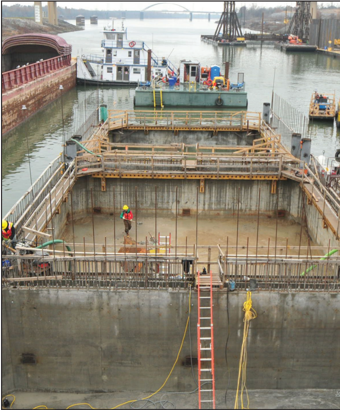
Figure 23. First three cofferdams in place, partially filled with inside concrete. Photo courtesy of Johnson Brothers Southland Holdings.
