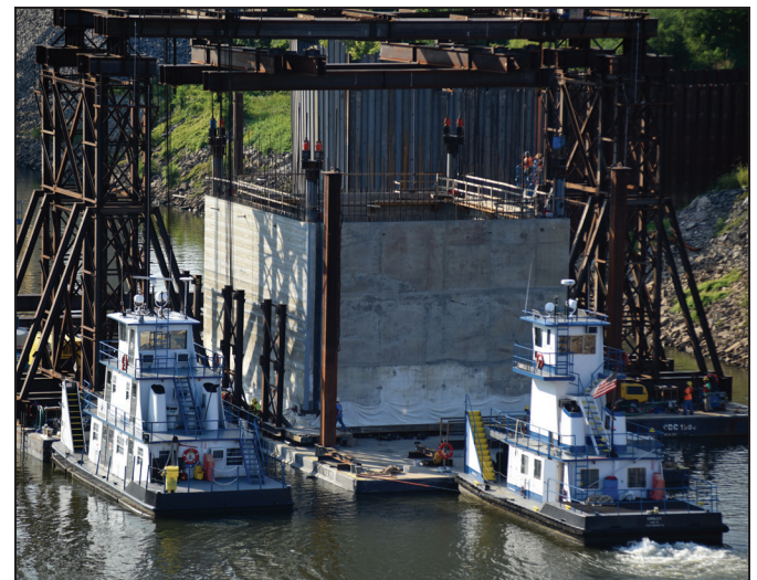
Figure 3. Towing the barge with the precast concrete cofferdam to the final location. Reproduced by permission from the U.S. Army Corps of Engineers.
