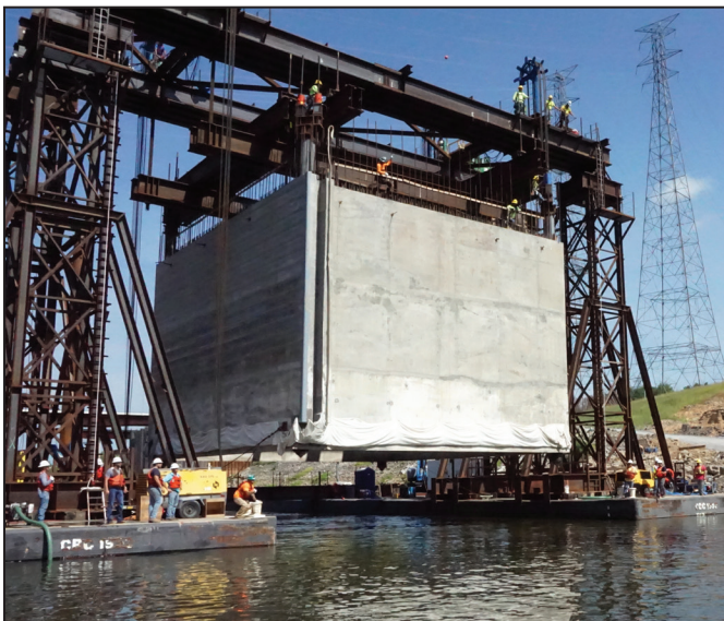
Figure 5. Lifting the precast concrete cofferdam. Reproduced by permission from the U.S. Army Corps of Engineers.
