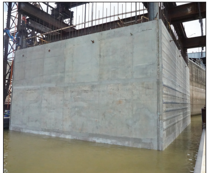
Figure 6. Precast concrete cofferdam placement in the river. Reproduced by permission from the U.S. Army Corps of Engineers.
