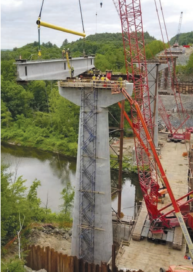
A 440-ton (400-tonne) crane places the first of the massive haunched precast concrete bulb-tee girder segments more than 130 ft (40 m) above the Williams River as part of a twin bridge replacement project on Interstate 91 in Rockingham, Vt. Courtesy of JP Carrara & Sons Inc.
