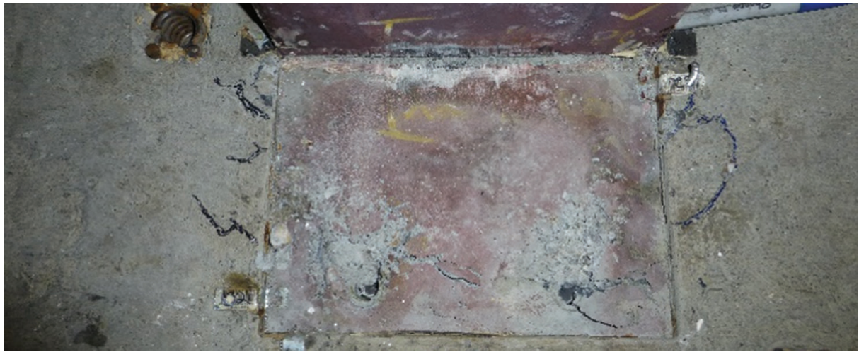
Figure 8. Lightly damaged concrete around north studs of specimen 2-0-0.92.
