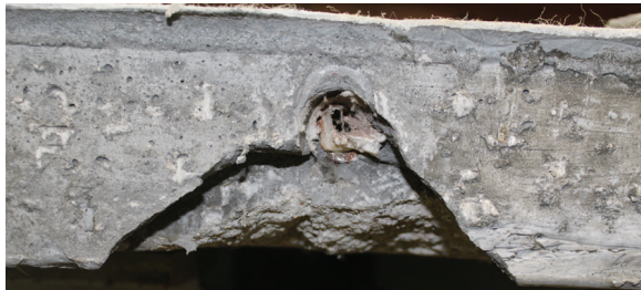
Concrete spalling from the bottom surface of the fixed panel
