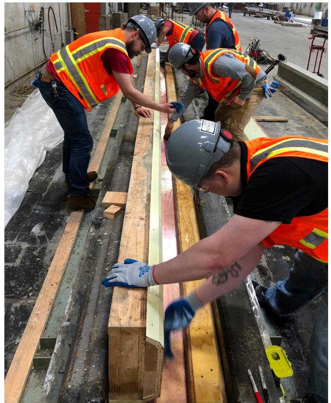
Saint Martin's University students constructing the form for their beam at Concrete Technology Corp. in Tacoma, Wash., for the Big Beam Contest. Courtesy of Jared Roschi.
