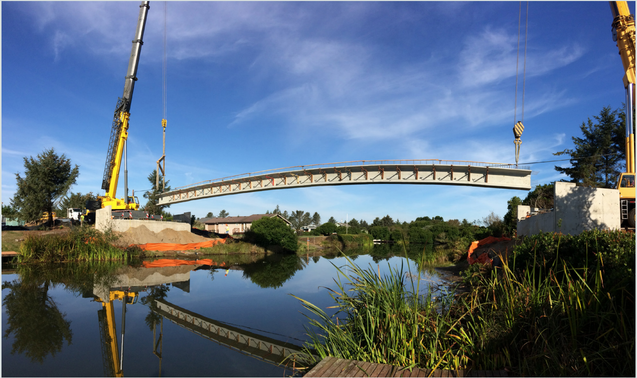
Figure 1. Precambered girder for the South Razor Clam Bridge in Ocean Shores, Wash. Courtesy of Concrete Technology Corp.
