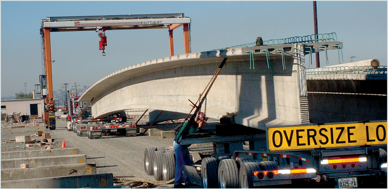
Figure 10. Precambered girder being prepared for transport to the Interurban Trail Pedestrian Bridge jobsite. Courtesy of Concrete Technology Corp.
