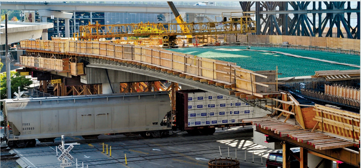
Figure 12. State Route 519 Royal Brougham Bridge girders precambered to provide vertical clearance for railroad tracks beneath the structure. Courtesy of Concrete Technology Corp.
