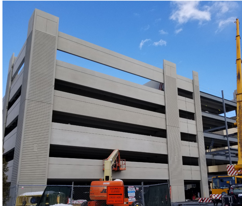
Blakeslee Prestress helped with this second parking structure at Cambridge Discovery Park in Cambridge, Mass., almost a decade after providing precast concrete for the first. The area had been built up more in the meantime, making access tighter. Courtesy of Blakeslee Prestress.
