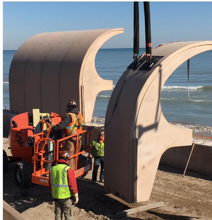
Workers install one of the 109 precast concrete segments that make up Northwestern University's precast concrete wave wall. Utility Concrete Products used column shoes with a threaded rod on the back side of the wall to help with setting and picking up the next segment. Courtesy of Utility Concrete Products LLC.
