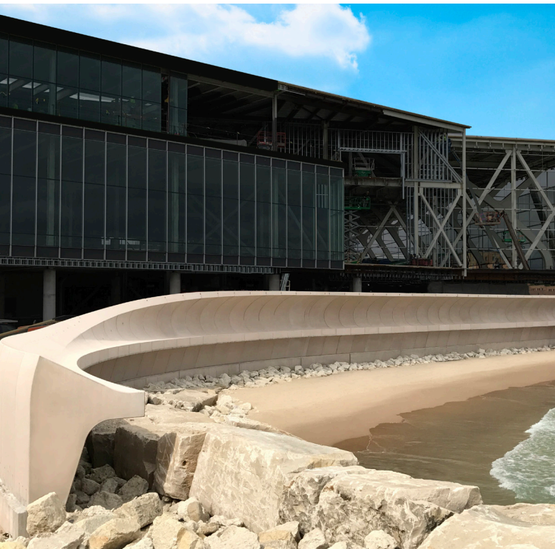
Northwestern University's precast concrete curving wave wall in Evanston, Ill., protects it from Lake Michigan's potentially destructive forces using precise placement of epoxy reinforcement, embedded stainless steel angles, and hot-dipped galvanized/epoxy connectors. Courtesy of Utility Concrete Products LLC.
