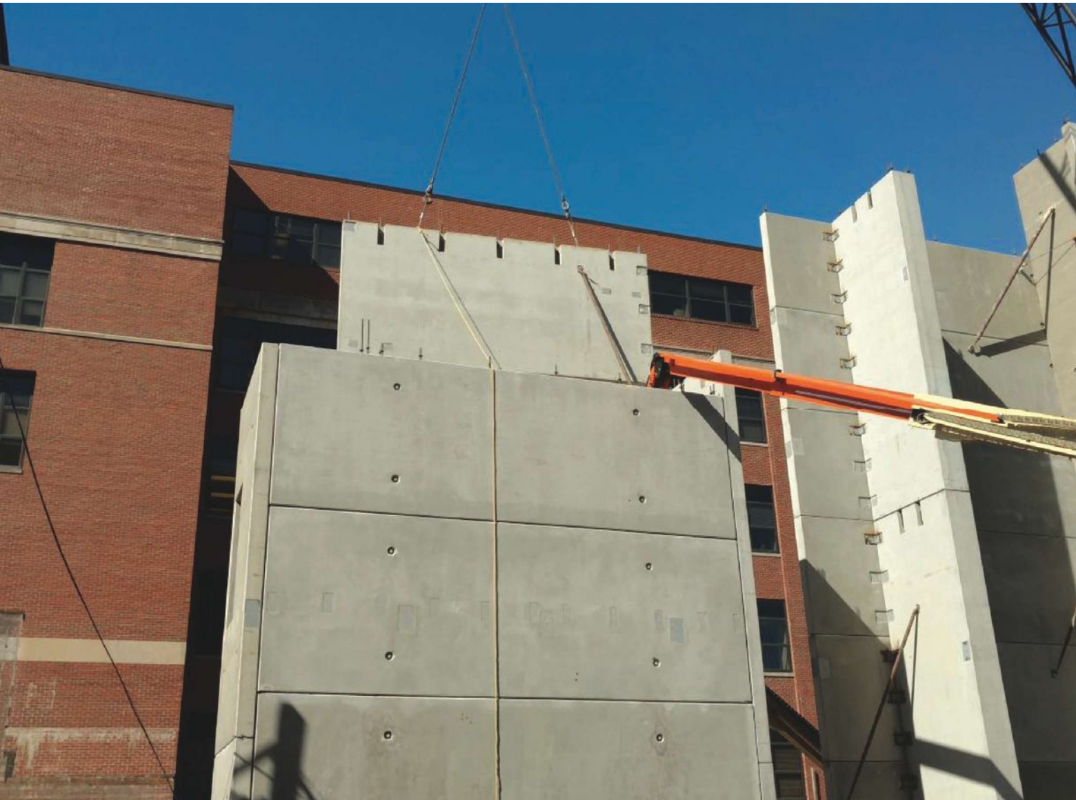
In 18 working days, 146 pieces were installed to construct the cores. Courtesy of Kerkstra Precast.
