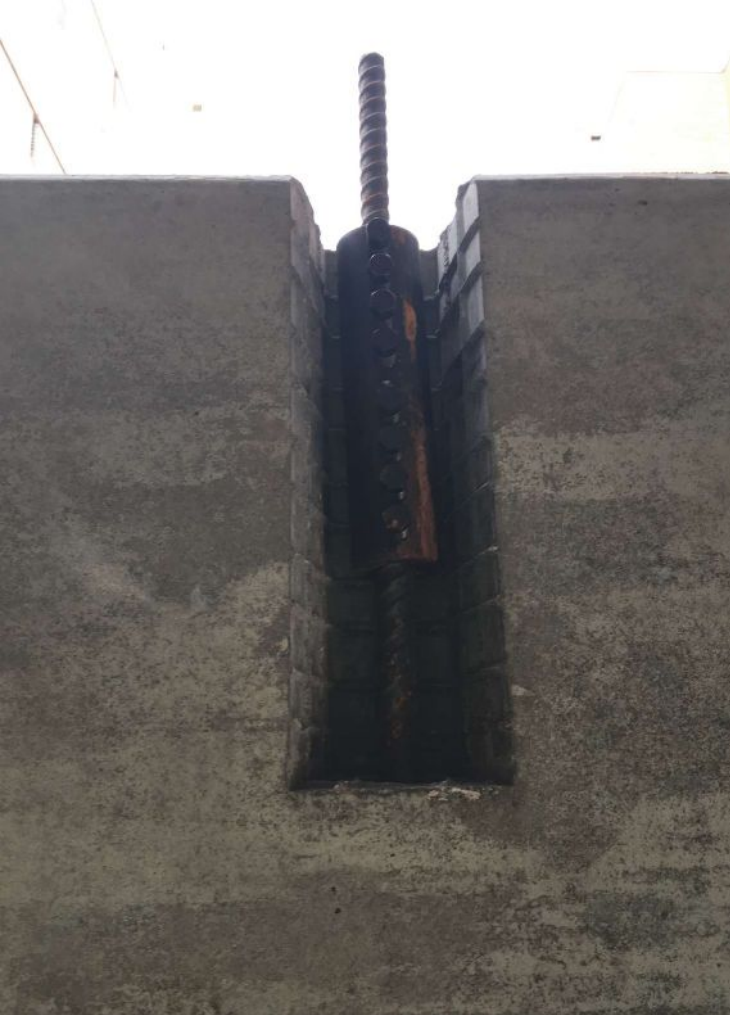
Bolted mechanical splice pockets in the precast concrete panels had to be filled with concrete later. Therefore, the pockets required roughened surfaces to improve the bond between precast concrete and cast-in-place fill. Courtesy of Kerkstra Precast.
