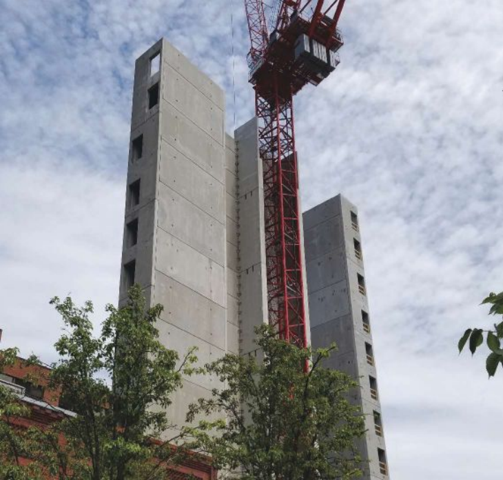
Precast concrete cores are shown during the construction of a 12-story-plus-basement dormitory in Ann Arbor, Mich. Courtesy of Kerkstra Precast.
