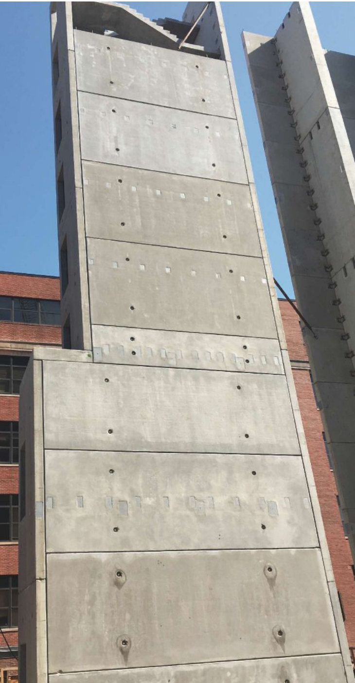
To enhance stability during erection, the precast concrete core was erected in a helical installation sequence pattern. Courtesy of Kerkstra Precast.
