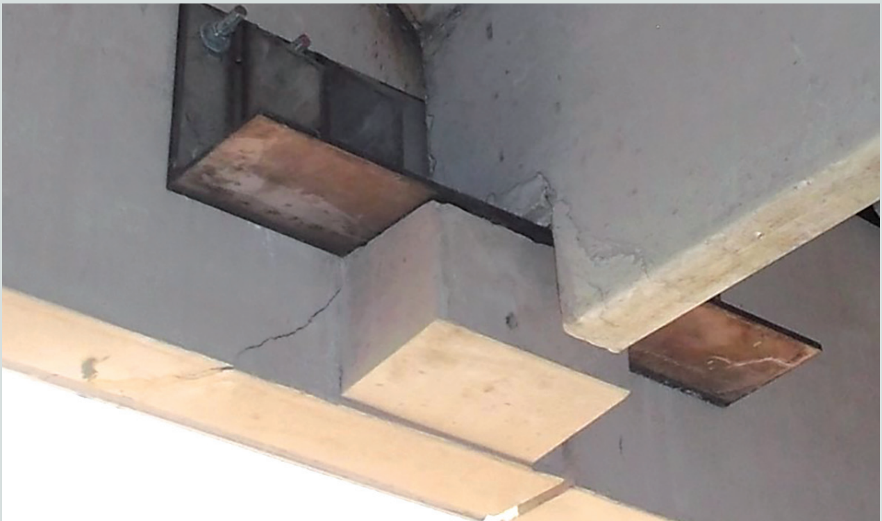
Figure 2. Distress in wall panel corbel with inadequate hanger reinforcement. Note: The steel angle was installed as a retrofit.
