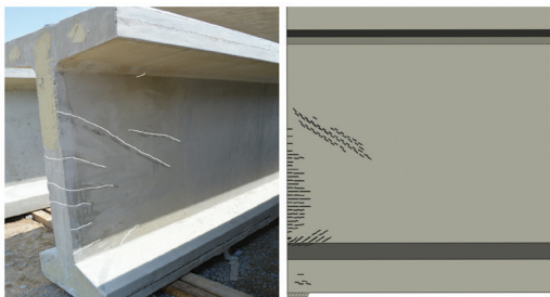
b) Comparison of observed and FEA cracking after detensioning
