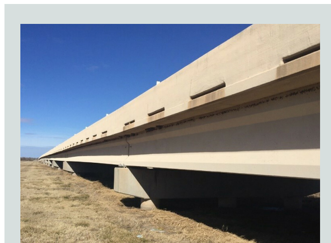
Figure 1. North Canadian River overflow structure, John Kilpatrick Turnpike, Okla., consisting of nineteen 103 ft 4 in. (31.5 m) spans in both northbound and southbound directions with Type IV girders spaced at 8 ft 9 in. (2.7 m) on center.
