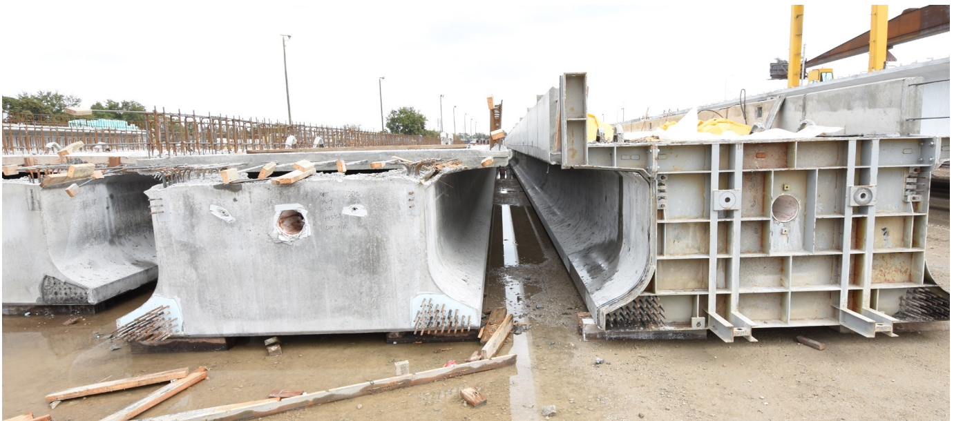
Pi girders, shown in the precasting yard, are being used to support the multiuse path bridge portion of the Pensacola Bay Bridge. Courtesy of WSP.
