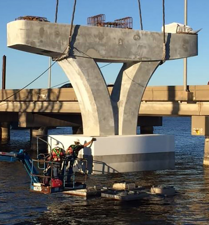
A one-piece V pier is set in the field for the Pensacola Bay Bridge. Courtesy of WSP.
