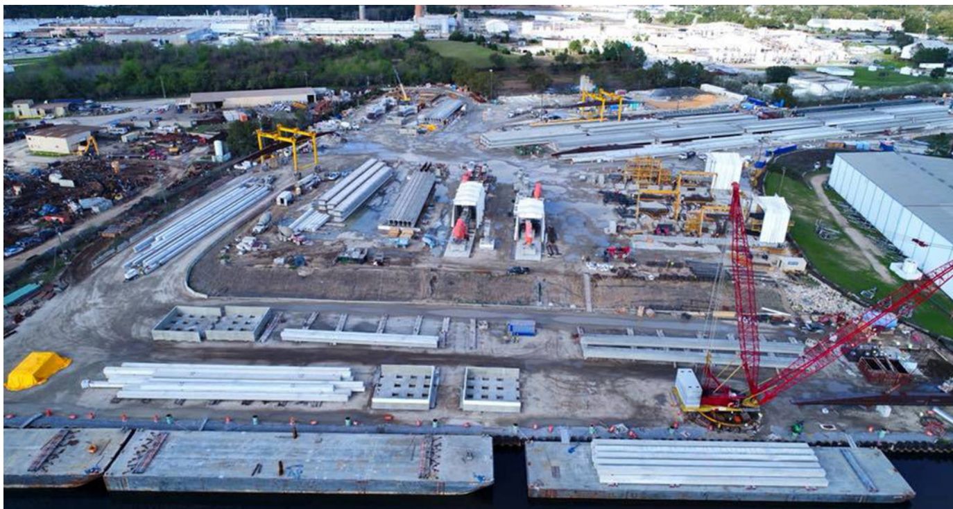
The precast concrete elements for the Pensacola Bay Bridge were fabricated at this on-site facility. Courtesy of WSP.
