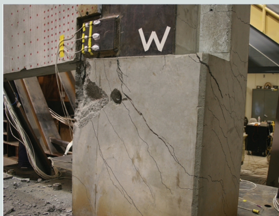
Special moment frame damage
