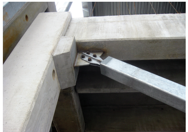
Typical upper connection of buckling-restrained brace to precast concrete beam and column.
