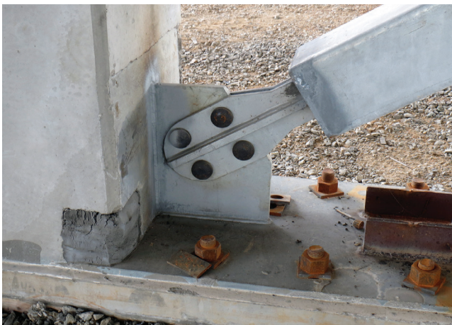
Typical lower connection of buckling-restrained brace to base plate and precast concrete column.
