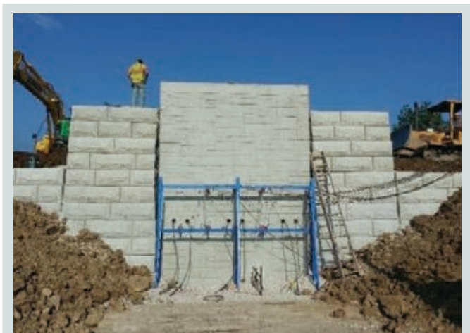
Figure 3. Front elevation of the totally prefabricated counterfort retaining wall system with wing walls.
