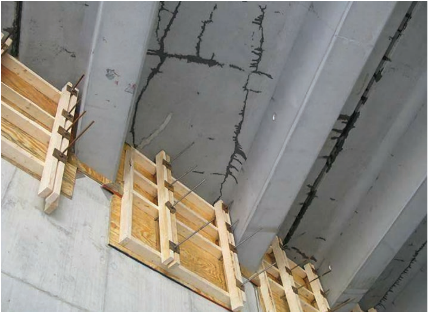
Figure 1. Flange bottom-face cracks on NEXT beam. Courtesy of Rita Seraderian, PCI Northeast.
