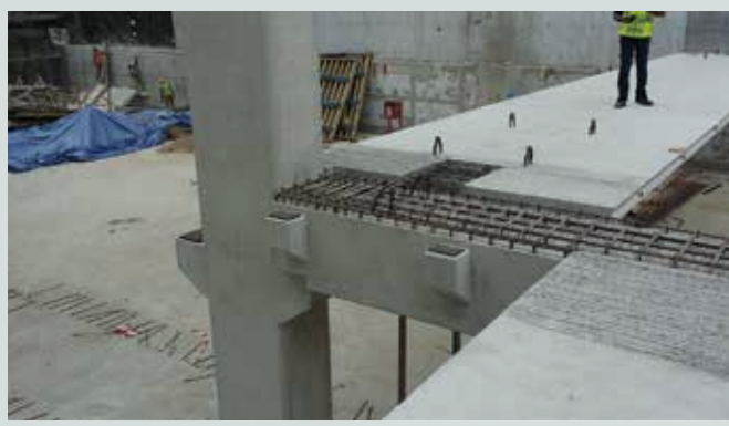
Figure 20. Box-beam slab being erected for underground parking structure in Abu Dhabi, United Arab Emirates.
