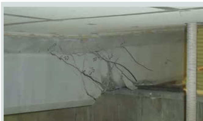
Figure 16. End shear failure and loss of strand bond.
