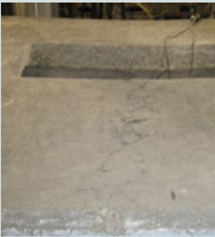
Concrete crushing in slab FO-O
