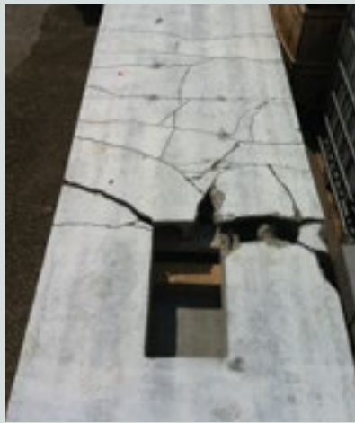
Slab SO-O at failure
