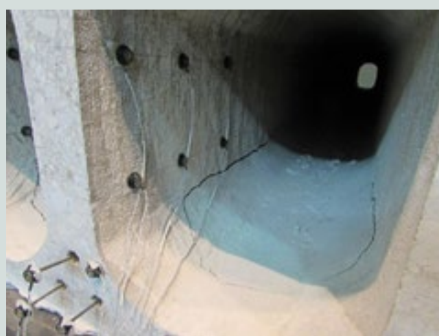
Figure 13. Horizontal cracking in interior web of 16 in. (410 mm) thick hollow-core slab (16-A1-W-3.0d).
