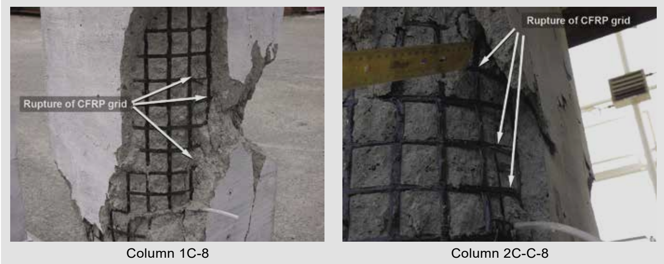
Figure 11. Rupture of CFRP grid strands at the conclusion of the test. Note: CFRP = carbon-fiber-reinforced polymer.
