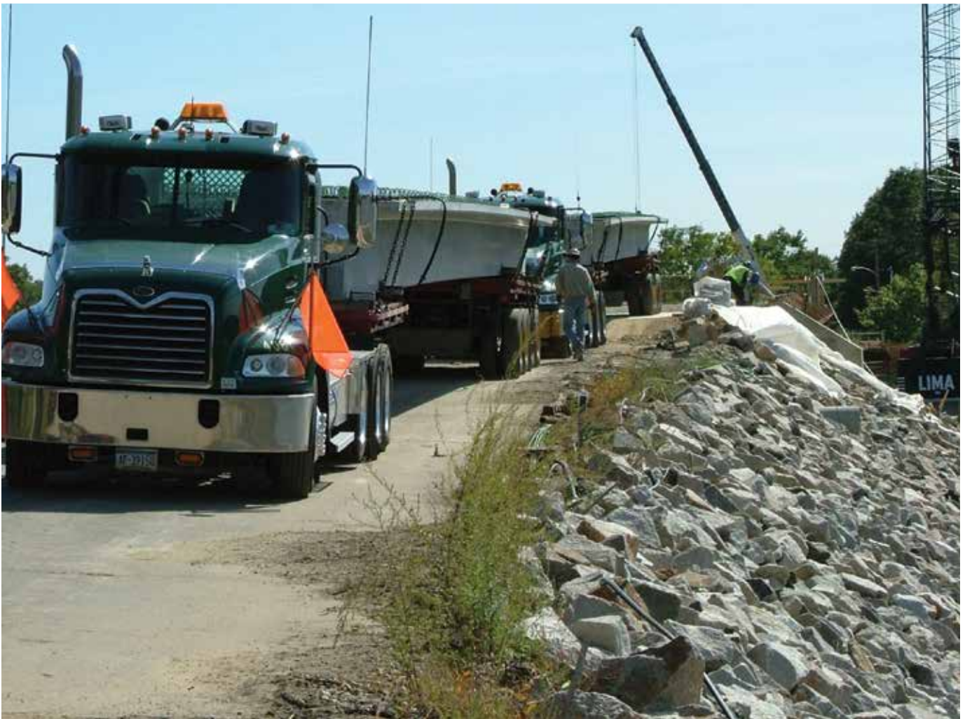
Figure 5. NEXT beam transport.
