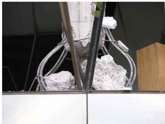
Figure 14. Reinforced concrete column with bar buckling and lack of confinement.
