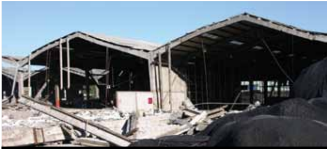
Figure 8. Precast concrete gable framed San José Fishery after the earthquake.
