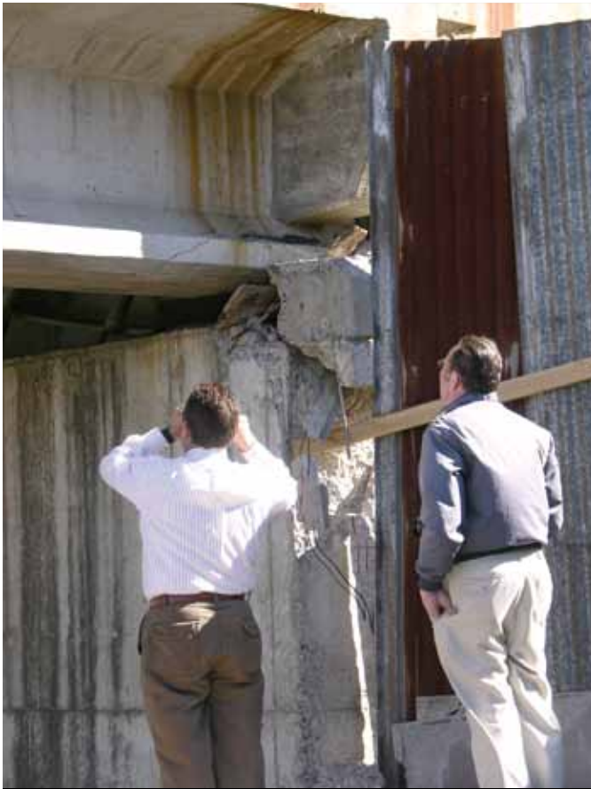
Figure 33. Failed stopper at the abutment of the Bio Bio River bridge, with a crack in the bottom of the girder.
