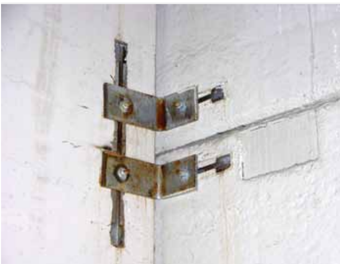
Figure 28. Slotted inserts to connect wall panels to concrete columns and the deformation of the slotted inserts due to the earthquake load.
