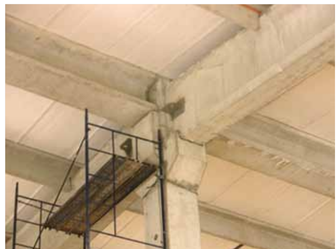
Figure 17. Wet-cast joint between girders and column in an industrial building that performed well during the earthquake.
