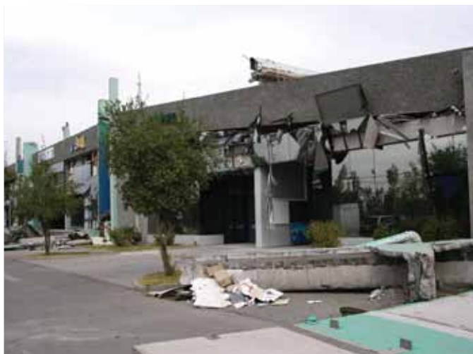
Figure 12. Front elevation of an office and warehouse building showing failed beam-column framing.
