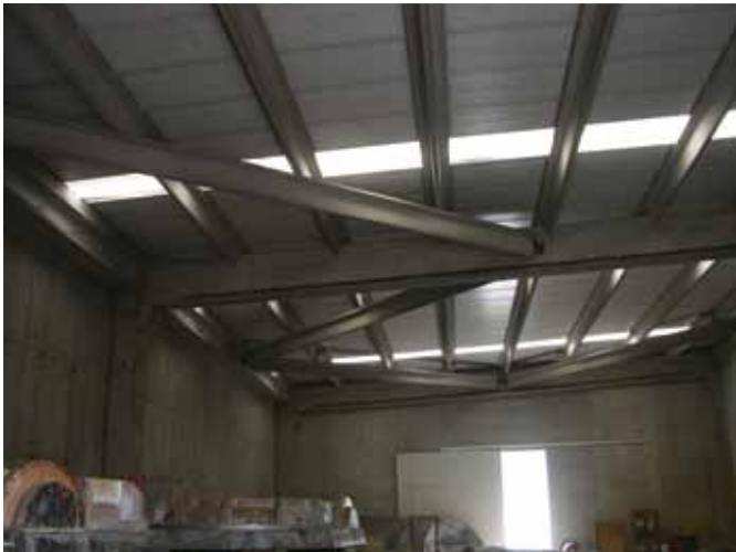
Figure 18. Diagonal precast concrete bracing for precast concrete girder roof framing in an industrial building that did not experience structural damage during the earthquake.
