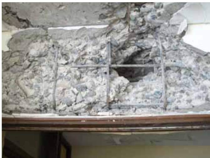
Figure 5. Damaged coupling beam in Viña del Mar, Chile.
