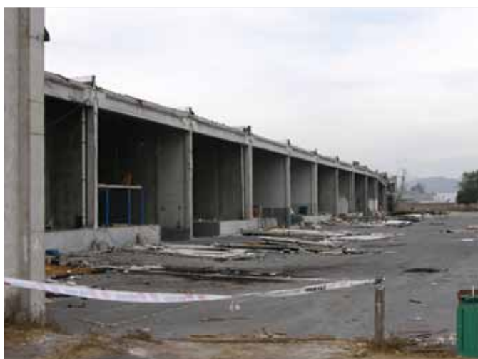
Figure 13. Rear elevation of the same office and warehouse building showing fallen exterior walls and exposed transverse walls and end columns.
