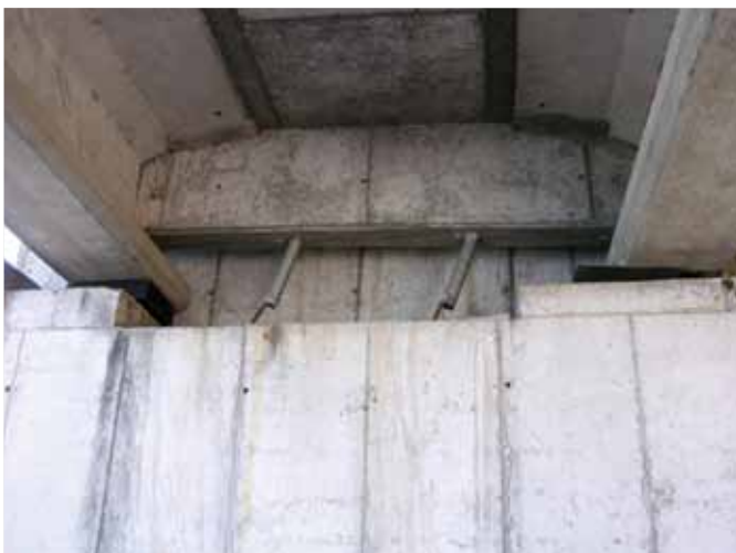
Figure 32. Lateral displacement due to earthquake forces of the Bio Bio River bridge with partial diaphragms and vertical restraint bars.
