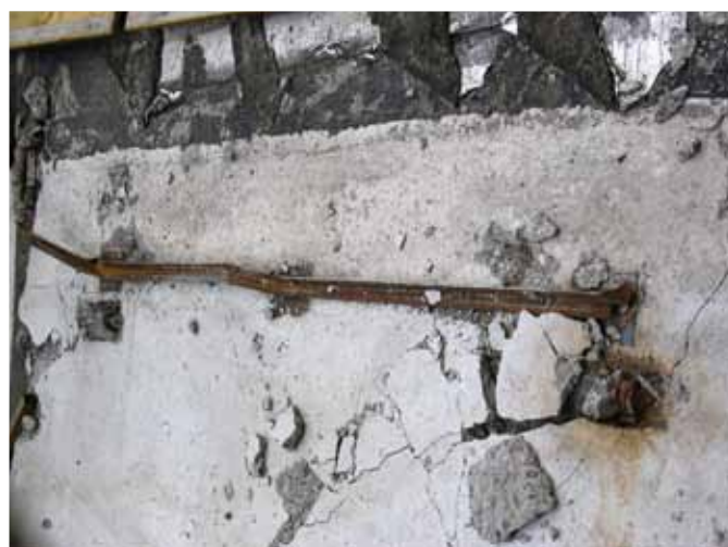
Figure 15. Bent and broken connection angle that failed to hold walls to edge beam at roof.
