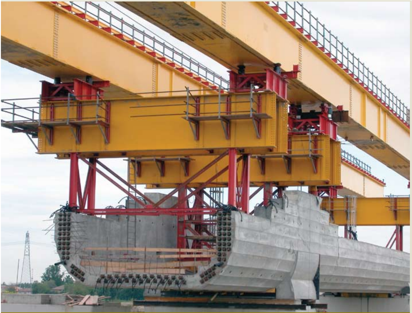
Figure 16. The buckling of the compression flange at the supports is due to the wrong operation.
