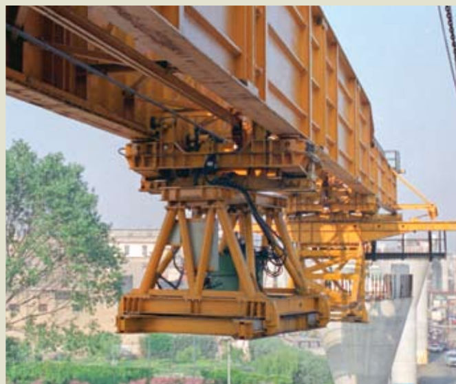
Figure 7. The friction launchers are suspended from the main girder.
