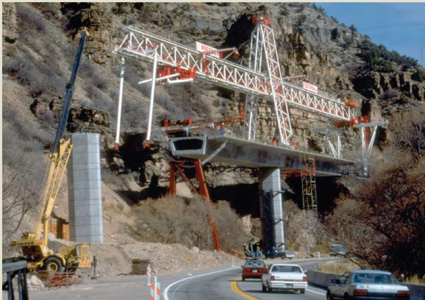
Figure 11. This single-upper-truss gantry is equipped with a deviation tower. Photograph courtesy of HNTB archive.
