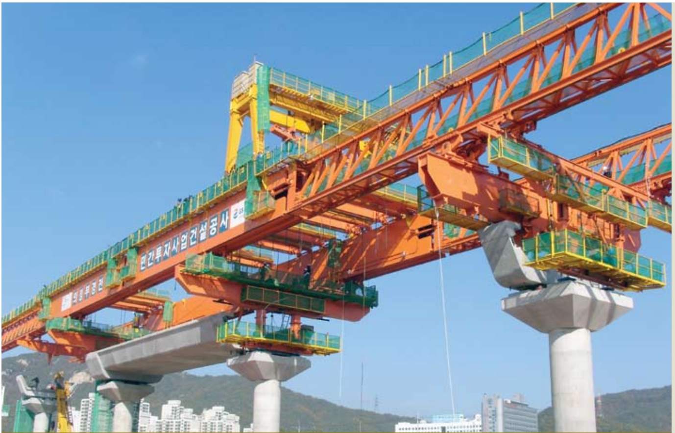
Figure 3. This shows a twin-upper-beam gantry with support cross beams. Photograph courtesy of NRS.
