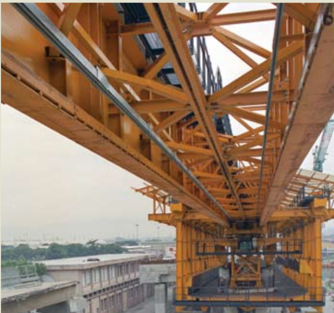
Figure 5. Lateral bracing of a single-upper-beam gantry in a movable scaffolding system configuration connects the plate girders along their entire length.
