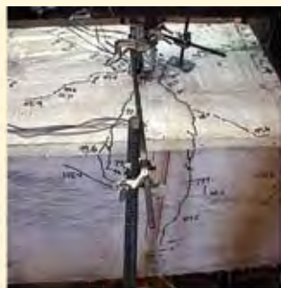
Splitting cracks near fracture of reinforcing bar VD03
