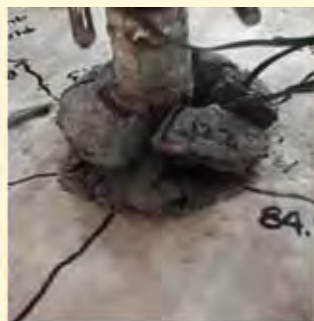
Pullout failure of VD04
