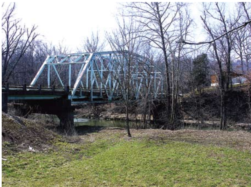
Old, deteriorated, steel-beam truss bridge over the Little Scioto River.
