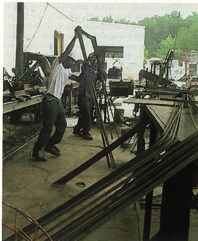
Fig. 4. Before spending large sums of money on an automated cutting and bending machine, correct the source of most waste with improved material flow and standardized procedures.
