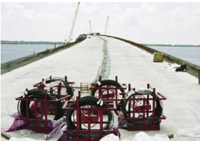
Fig. 20. The overall length of the spliced girder unit, 1180 ft (360 m), complicated the installation of the post-tensioning tendons.
