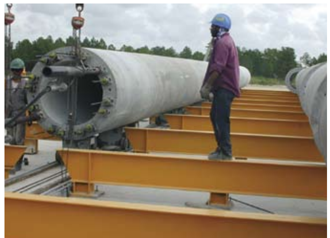
Fig. 16. Because of the size of the project, it was important to fabricate precast concrete elements in advance of construction.
