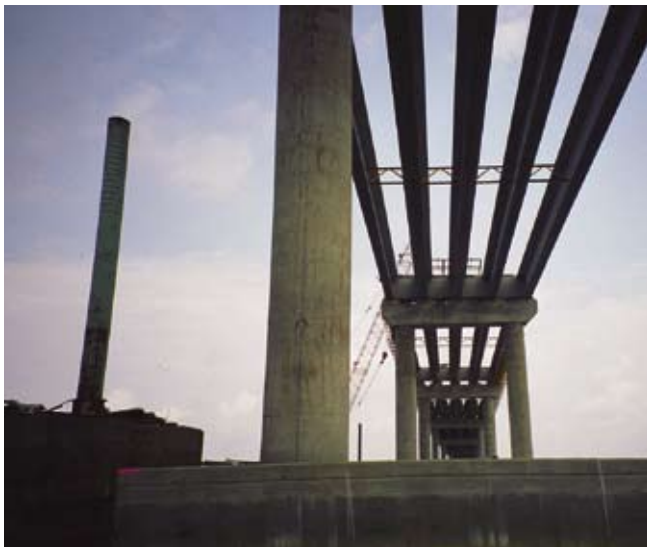
Fig. 12. As viewed from the bridge foundation, five lines of prestressed concrete girders were designed for the St. George Island Bridge high level and main channel sections.
