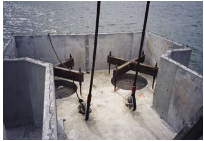
Fig. 18. Precast concrete footing forms were fabricated to account for the battered piles through the use of circular openings.
