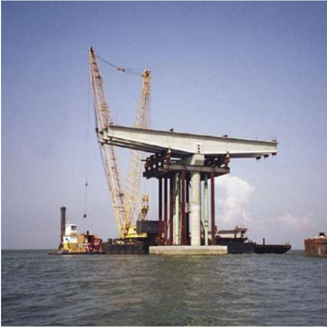
Fig. 19. Temporary shoring towers eliminated the need to drive temporary piles at the bridge piers.
