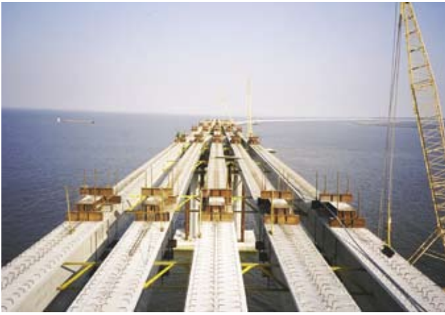
Fig. 5. St. George Island replacement bridge under construction prior to post-tensioning operations in the main channel span over the Intracoastal Waterway.
