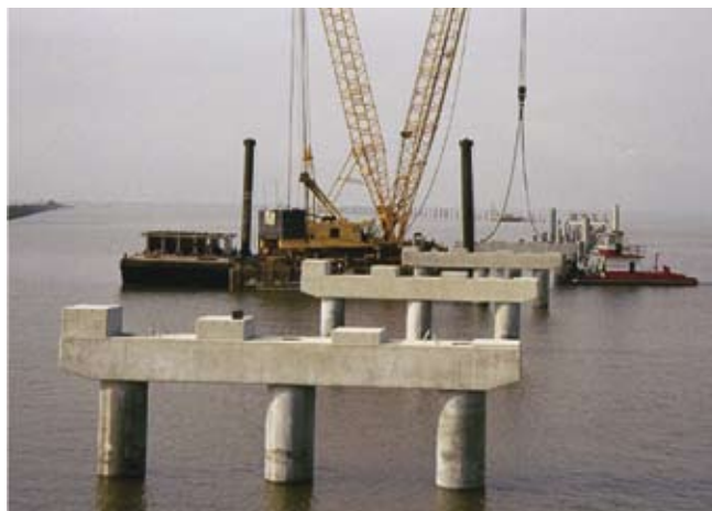
Fig. 9. Erection of precast concrete bent pile caps at the bridge construction site.
