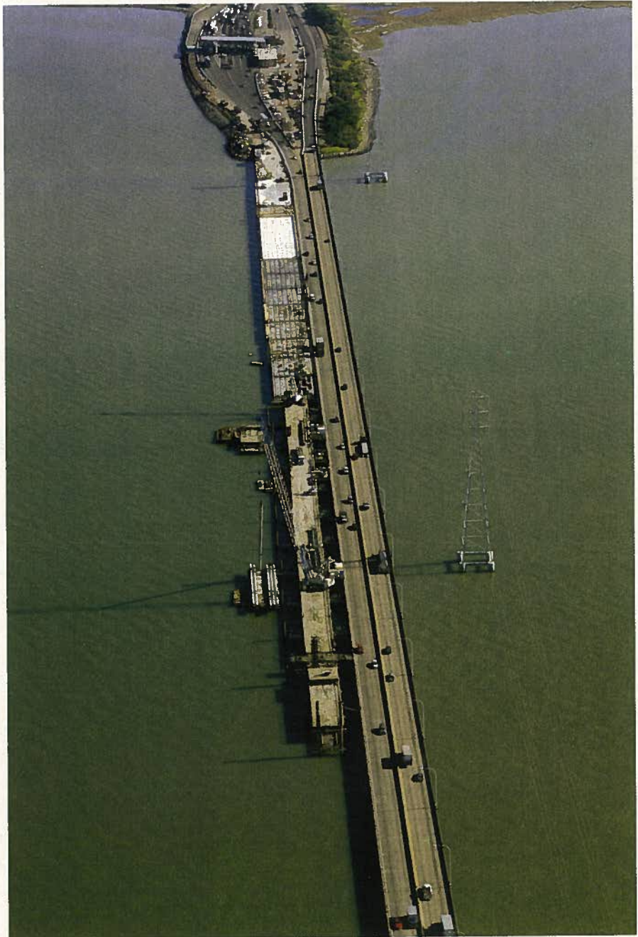
Fig. 23. Aerial view of the bridge widening under construction. (Courtesy of CALTRANS District 4 Photography Department)
