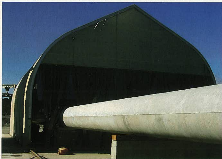
Fig. 17. Piles are loaded into the coating area prior to rolling the nested building enclosure into place over the piles. (Courtesy of Pomeroy Corporation)
