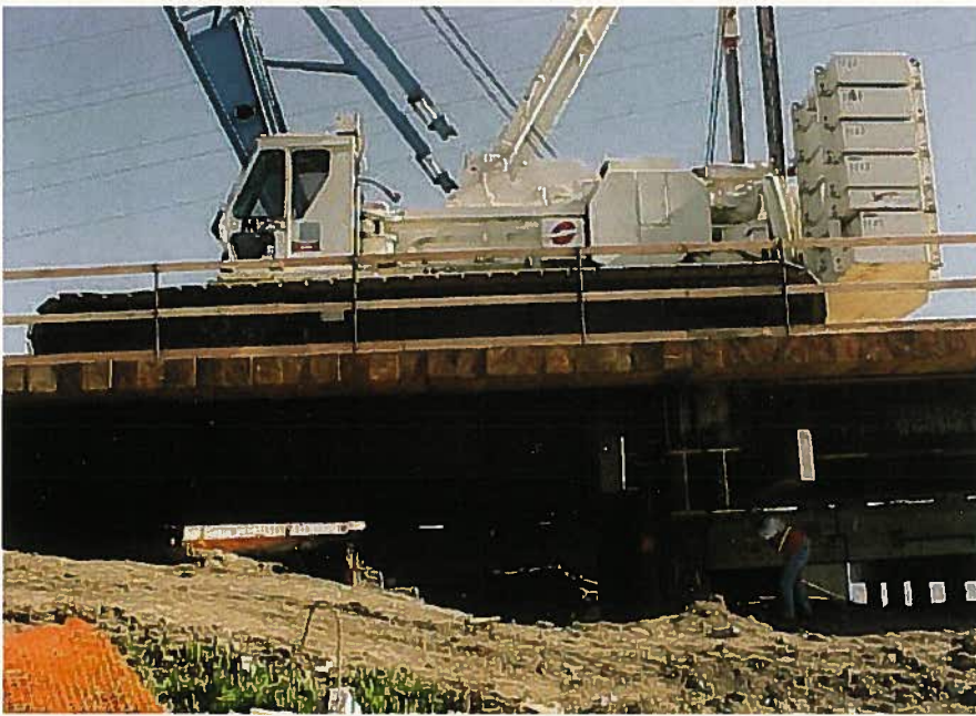
Fig. 19. Work platform supports crawler-mounted erection crane with counterweights. (Courtesy of Balfour Beatty Construction)
