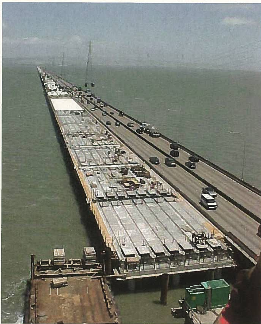
Fig. 3. Construction under way with temporary work platform adjacent to the existing bridge. Barge delivery of precast concrete components and a movable work trestle allowed traffic to flow uninterrupted on the old bridge. (Courtesy of Balfour Beatty Construction)
