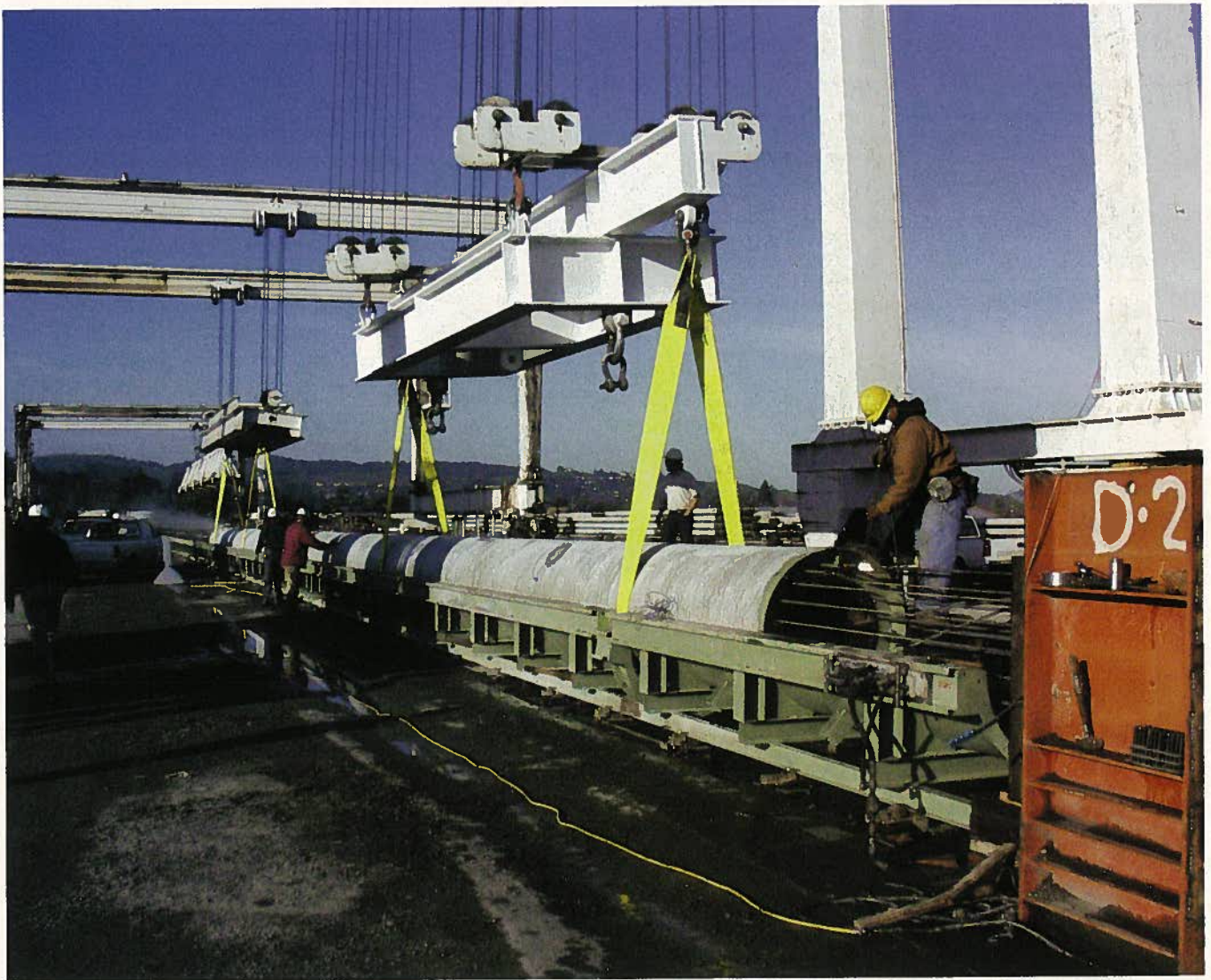
Fig. 7. Pile being removed from the form using slings and drop-out sections in the forms to eliminate the need for lift hooks. Lift hooks, even after removal and patching, could have presented potential ingress of saline water and subsequent pile reinforcing corrosion. (Courtesy of Pomeroy Corporation)
