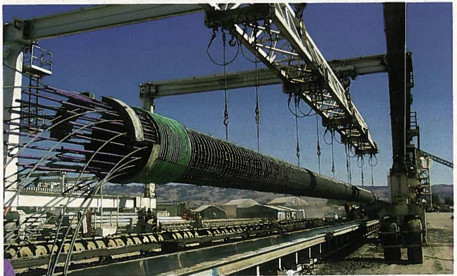
Fig. 8. Completed pile cage being lowered into the form at Pomeroy's precasting facilities in preparation for casting. Note the prestressing strand and the collapsible inner core form in place and lifted out as a single unit. (Courtesy of Pomeroy Corporation)
