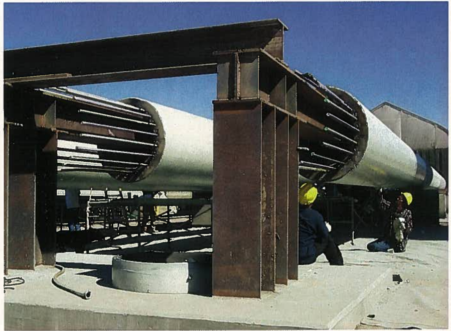
Fig. 18. Cylinder piles on custom-made steel supports that allow the polyurea coating to be applied to the full pile surface without having to turn or move the product. (Courtesy of Pomeroy Corporation)
