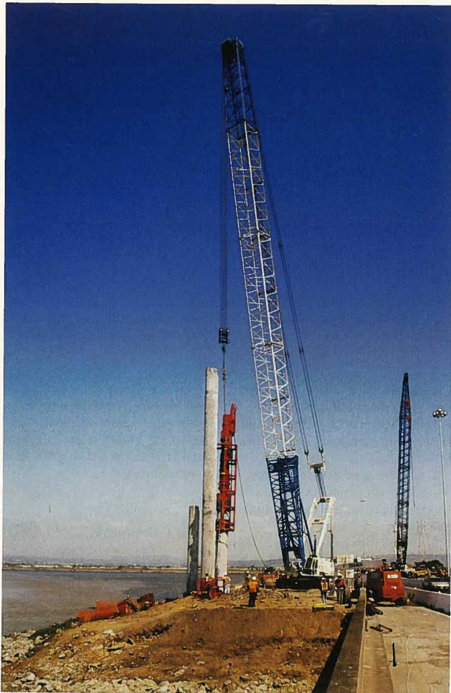
Fig. 22. Piles were located by GPS and template. After spotting, the pile was released and would run 40 ft (12 m) into the bay mud under its own weight. The driving hammer was then used to drive the pile to elevation. (Courtesy of Balfour Beatty Construction)
