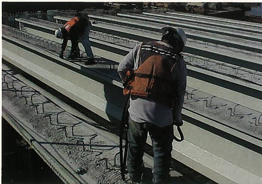
Fig. 13. Erection crew placing the rubber strip on top of the girder curb. This system supported the precast concrete flat slabs. (Courtesy of Balfour Beatty Construction)
