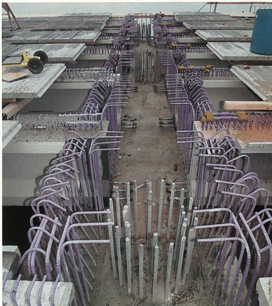
Fig. 14. Pile-cap connection immediately prior to field installation of reinforcement and placement of CIP concrete to secure the cap to the pile. Note top of precast pile and vertical pile reinforcement extending through the opening of the precast cap. (Courtesy of Balfour Beatty Construction)
