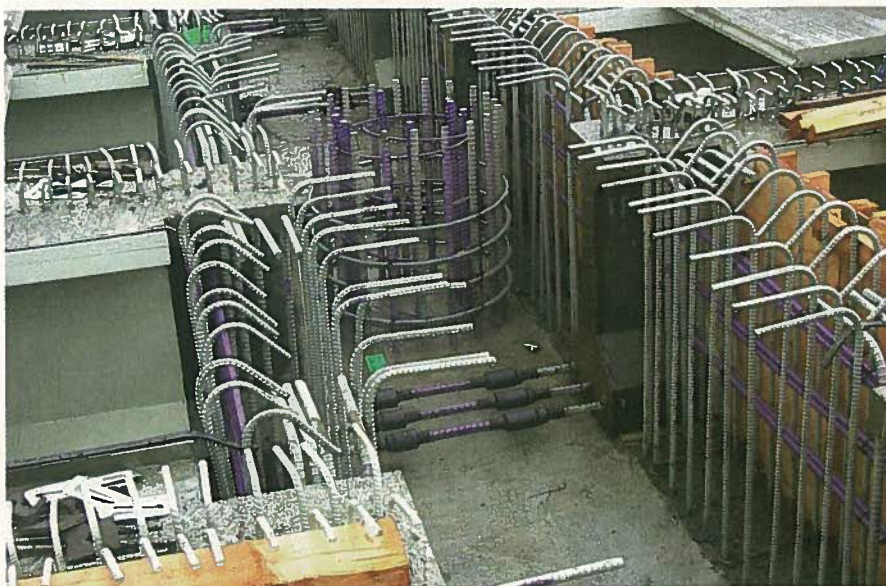
Fig. 11. Portion of the pier cap reinforcing steel above the extended rebar of a pier, just prior to the installation of the cap reinforcing steel. Note the mechanically coupled reinforcement extending from the bottom portion of each girder for positive moment forces at the bent. (Courtesy of Balfour Beatty Construction)
