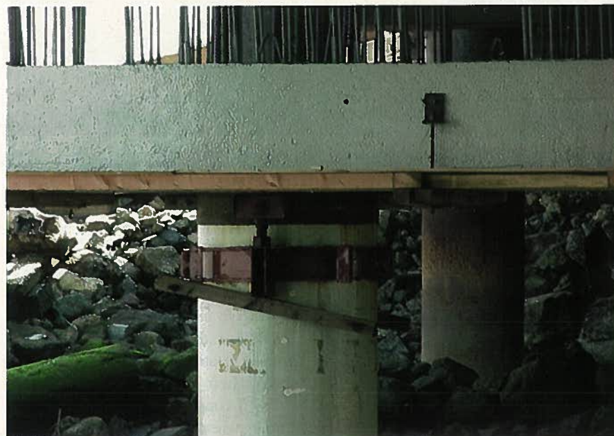
Fig. 15. A friction collar was used to temporarily support the precast caps. The collar remained in place until the precast cap was permanently attached to the piles with field-installed rebar and a CIP pour. (Courtesy of Balfour Beatty Construction)
