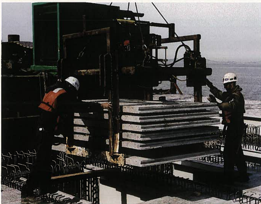
Fig. 20. Hoisting of precast deck panels with panel placing machine during construction. Ten precast concrete deck panels were used in each span. (Courtesy of Balfour Beatty Construction)
