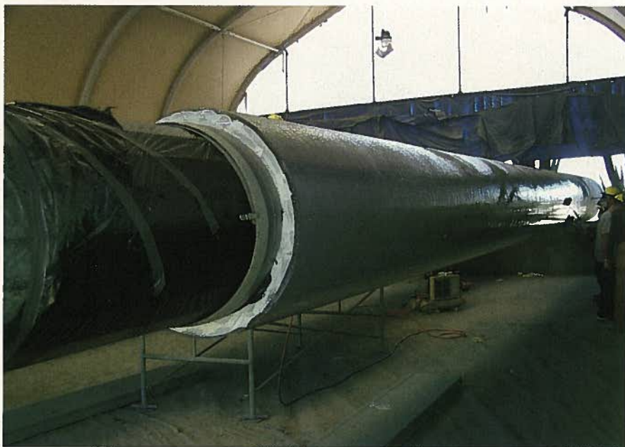
Fig. 16. Climate-controlled building protects bridge piles during polyurea coating application at the Pomeroy plant. (Courtesy of Pomeroy Corporation)
