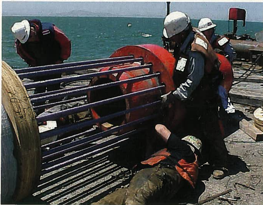
Fig. 10. The crew installing the pile-driver follower over precisely positioned steel dowel bars extending from the top of a pile. The follower allows the energy from the pile driver hammer to be delivered to the top of the pile itself while simultaneously protecting the vertical pile reinforcement. Note the wooden pile driving cushion has already been installed. (Courtesy of Balfour Beatty Construction)
