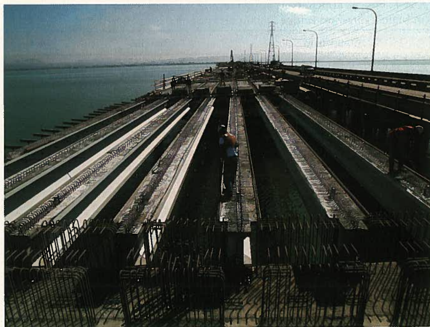
Fig. 12. End view of bridge widening construction reveals the eight bulb-tee girder layout beneath the precast deck slabs. (Courtesy of CALTRANS District 4 Photography Department)
