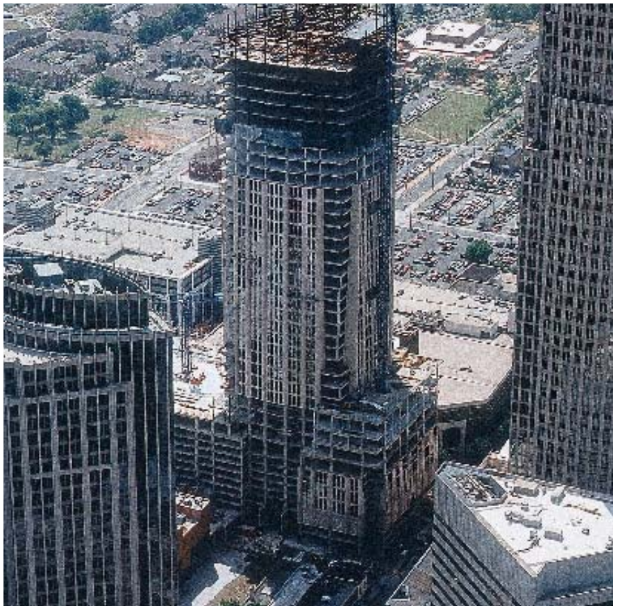
Fig. 5. With a sidewalk-to-sidewalk footprint, the urban site limitations meant little storage space and maneuvering room for equipment and construction trades.
