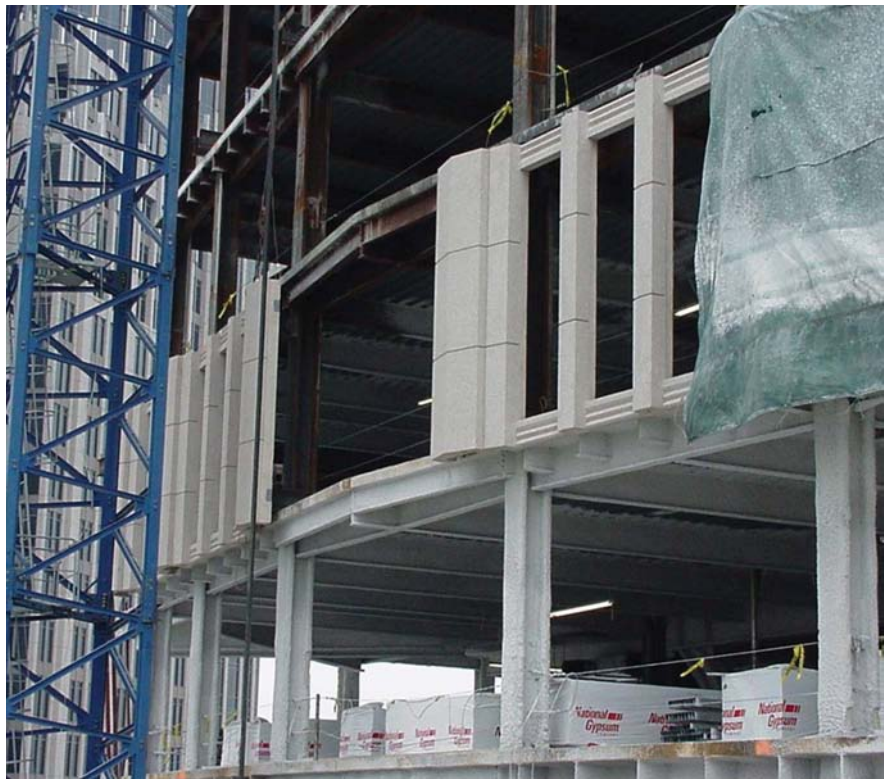
Fig. 12. The precaster and designers worked together to produce an innovative window unit panel that allows the architectural element to span from floor to floor, thereby reducing the total number of panels for erection.
