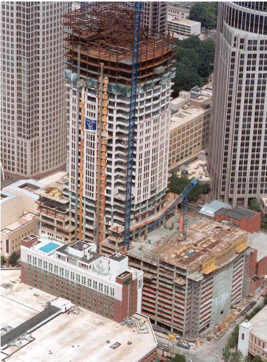
Fig. 14. View from the IJL Financial Center, showing construction of the lower levels of the Hearst Tower.
