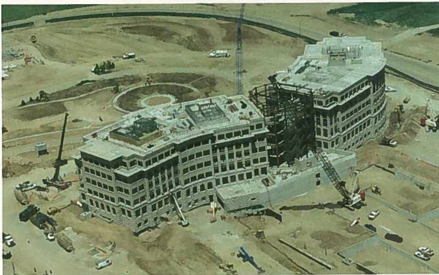
Fig. 4. Two dogleg-shaped units turned 180 degrees connect at a central glass atrium with steel framing.
