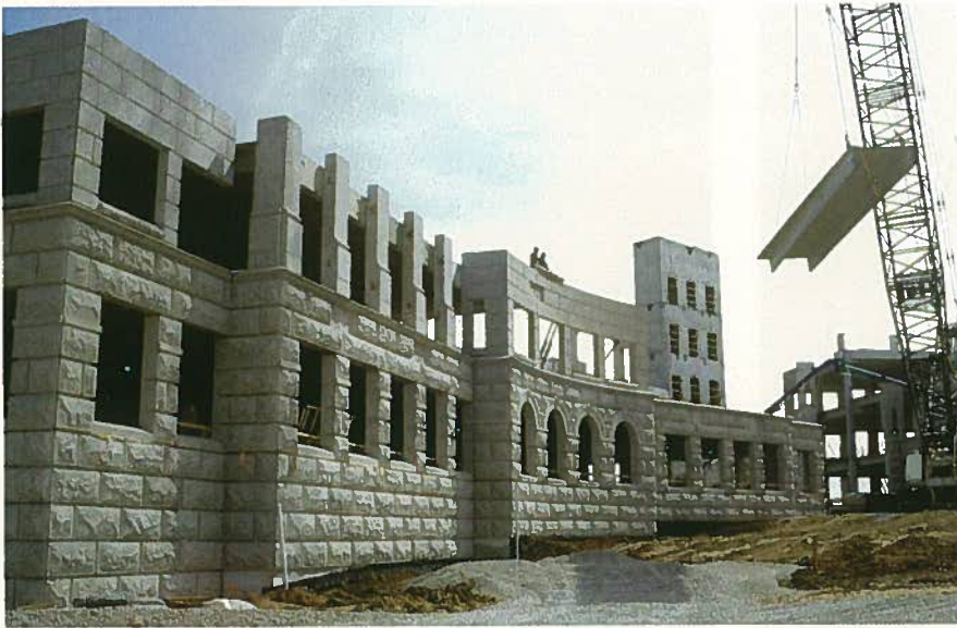
Fig. 14. Two 250 ton Manitowoc cranes were used to erect the precast elements at the central rotunda of the Starz Encore Headquarters. Heavier precast panels weighed as much as 58,000 lbs (26000 kg).
