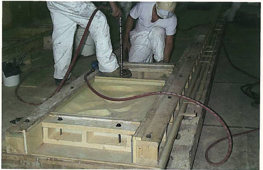
Fig. 8. Innovative filler pieces or “soaps” were used to create imperceptible connections between precast panels.
