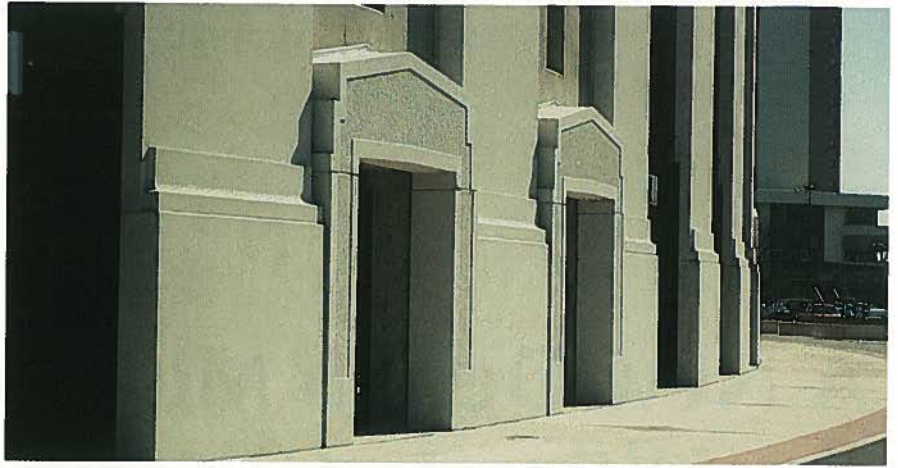
Fig. 20. Entrance portals were given a bush-hammered finish to work in aesthetic harmony with the older existing cast-in-place concrete.
