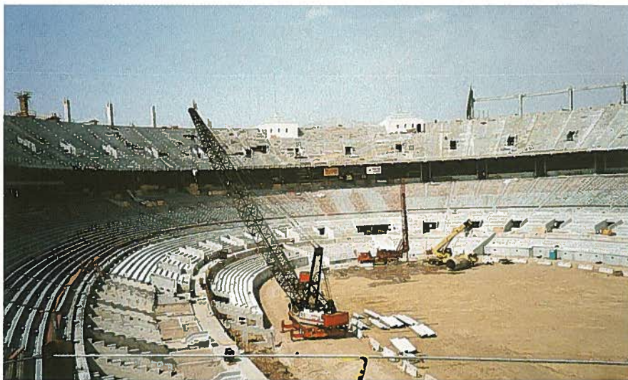
Fig. 10. New playing surface, excavated down 14 ft (4.3 m), places the playing field almost 6 ft (2 m) below the groundwater table.
