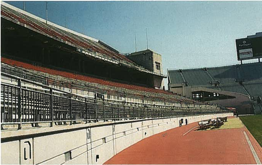
Fig. 16. Architectural precast concrete fascia walls at playing level provided owner-pleasing detailing of the OSU block "O" logo.
