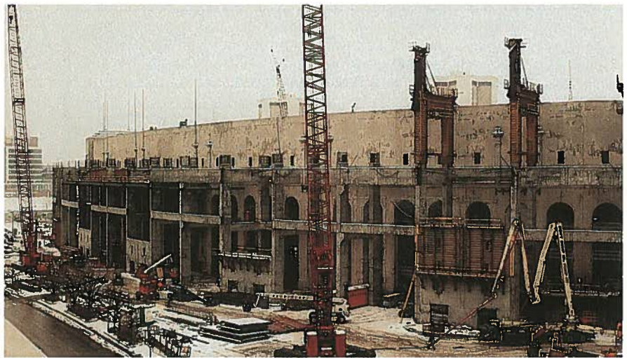
Fig. 13. Cast-in-place concrete columns and platforms provide structural support for precast expansion for the new Upper C Deck.
