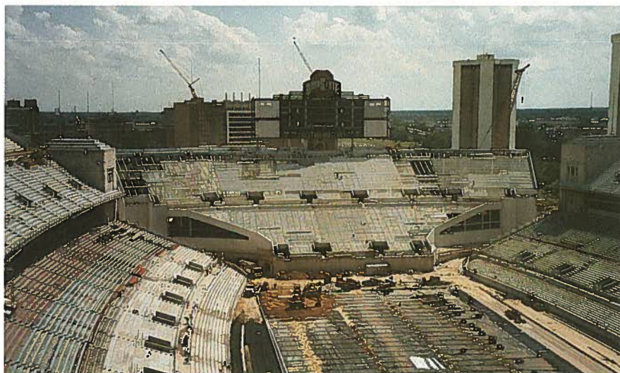
Fig. 11. Once the initial construction for the engineered turf drainage system began, no construction equipment was permitted on the stadium infield.
