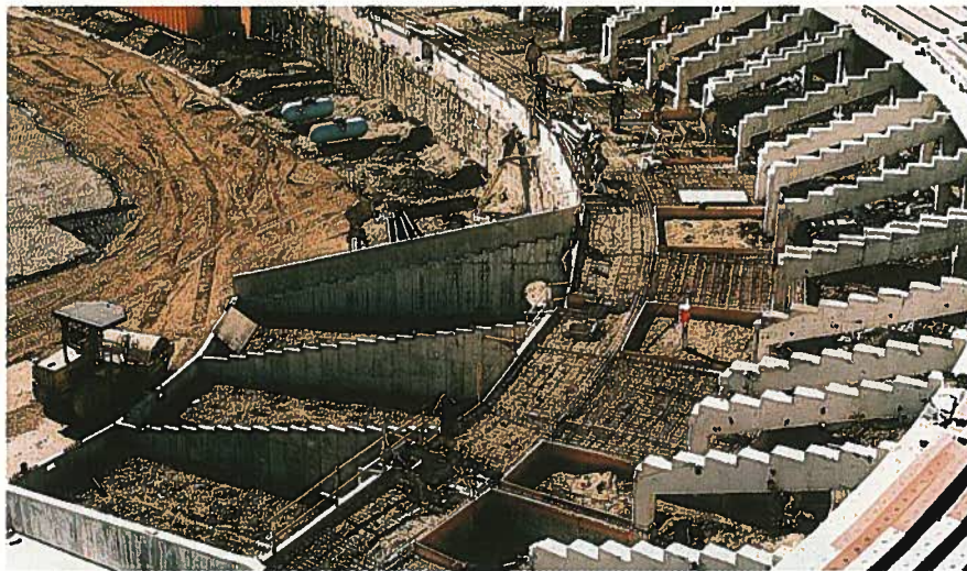
Fig. 8. Erection of the structural precast concrete raker beams at the excavated Lower AA Deck.
