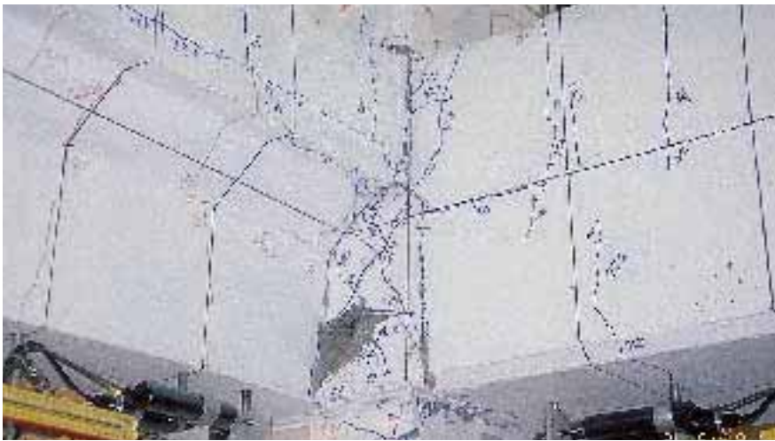
Fig. 9a. Joint damage of Specimen J2 at design drift of 2 percent, east-west direction.
