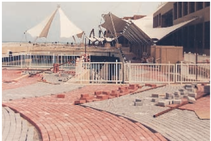
Fig. 16. Precast concrete pavers in red and gray tones were installed on all walkways in a scallop pattern to add visual interest and set off the complex's landscaping.
