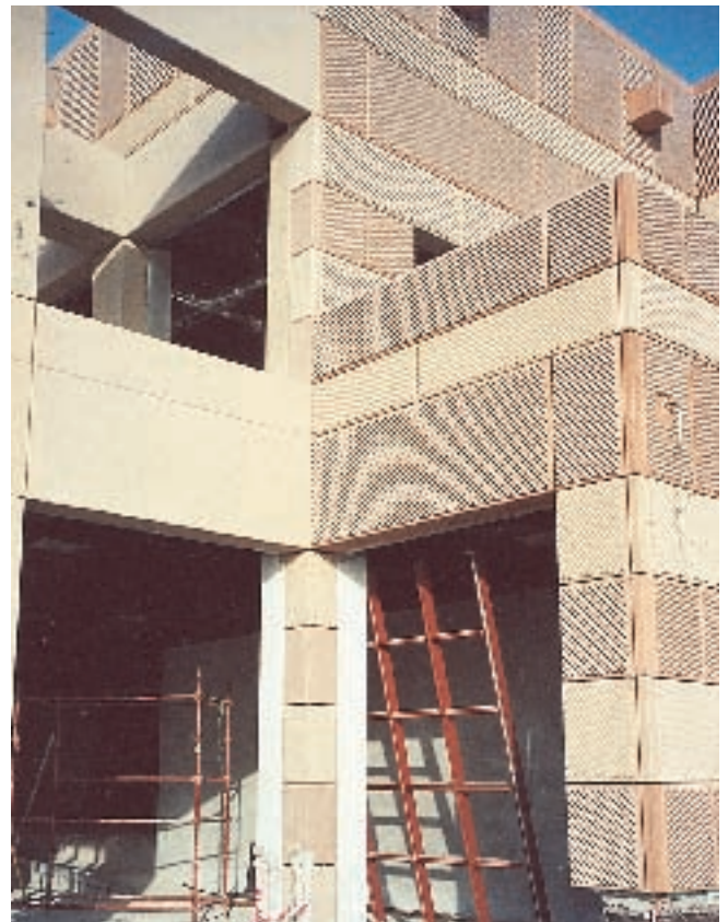
Fig. 7. Precast concrete panels with sand-colored buff and light terra cotta coloring contrast with lightly sandblasted panels to create visual interest.
