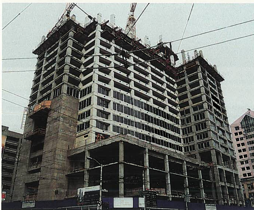
Fig. 20. Progress view of precast frame erection. Photo courtesy: Kwan Henmi, Architecture and Planning.
