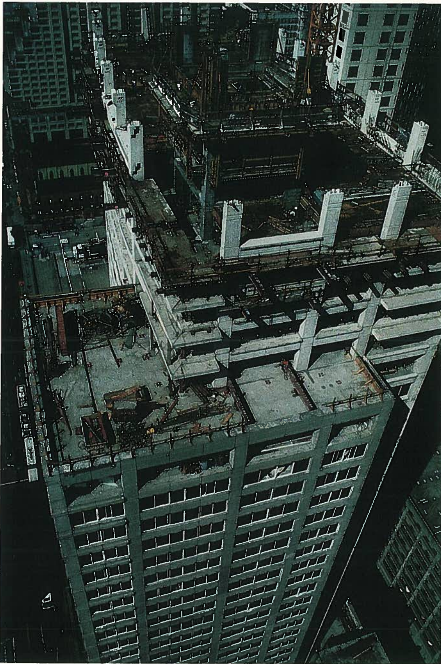
Fig. 21. Erection of precast perimeter frames nearing top of building. Photo courtesy: Kwan Henmi, Architecture and Planning.
