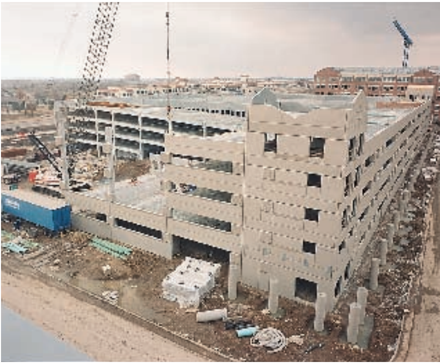
Fig. 14. Erection of one of the parking structures. Note the ribbed column covers.
