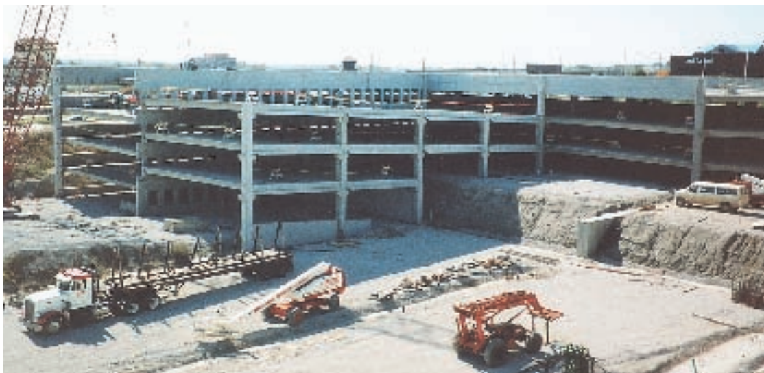
Fig. 11. Variations in slope created some challenges in laying out the first floors of the structures.
