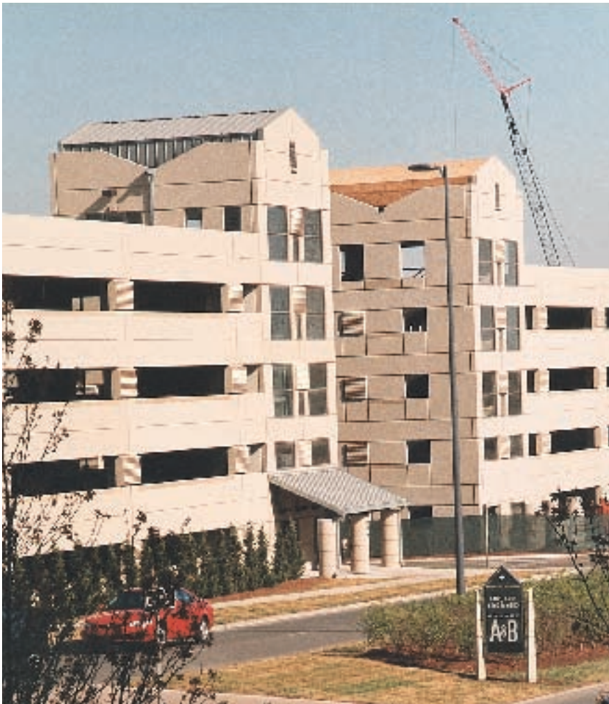
Fig. 2. Parking structures at Sprint's Worldwide Headquarters in Overland Park, Kansas, were designed with a simple style with a few decorative touches.
