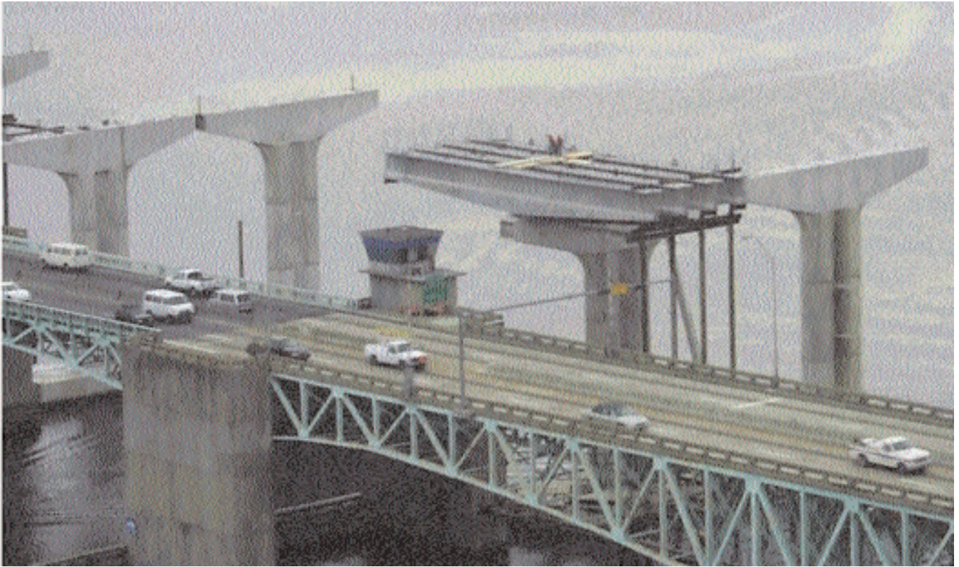
Fig. 15. Column pier with cantilevered haunched pier beam segments (Fuller Warren Bridge, Florida).
