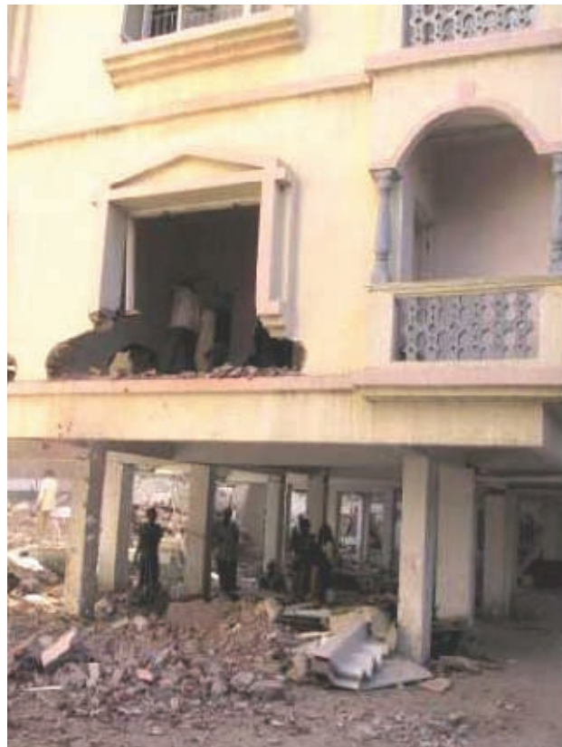
Fig. 6. Typical soft-story residential building. Courtesy: Tiziana Rossetto, Imperial College, London.
