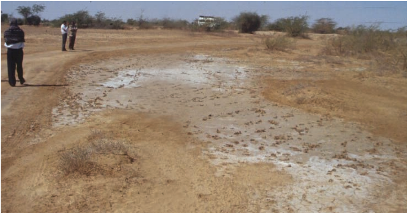
Fig. 4. Liquefaction caused by earthquake. Courtesy: MAE Center.
