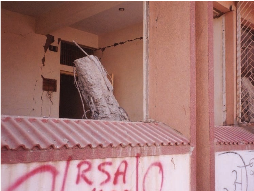
Fig. 9. Ground level column punching through floor slab of a building.
