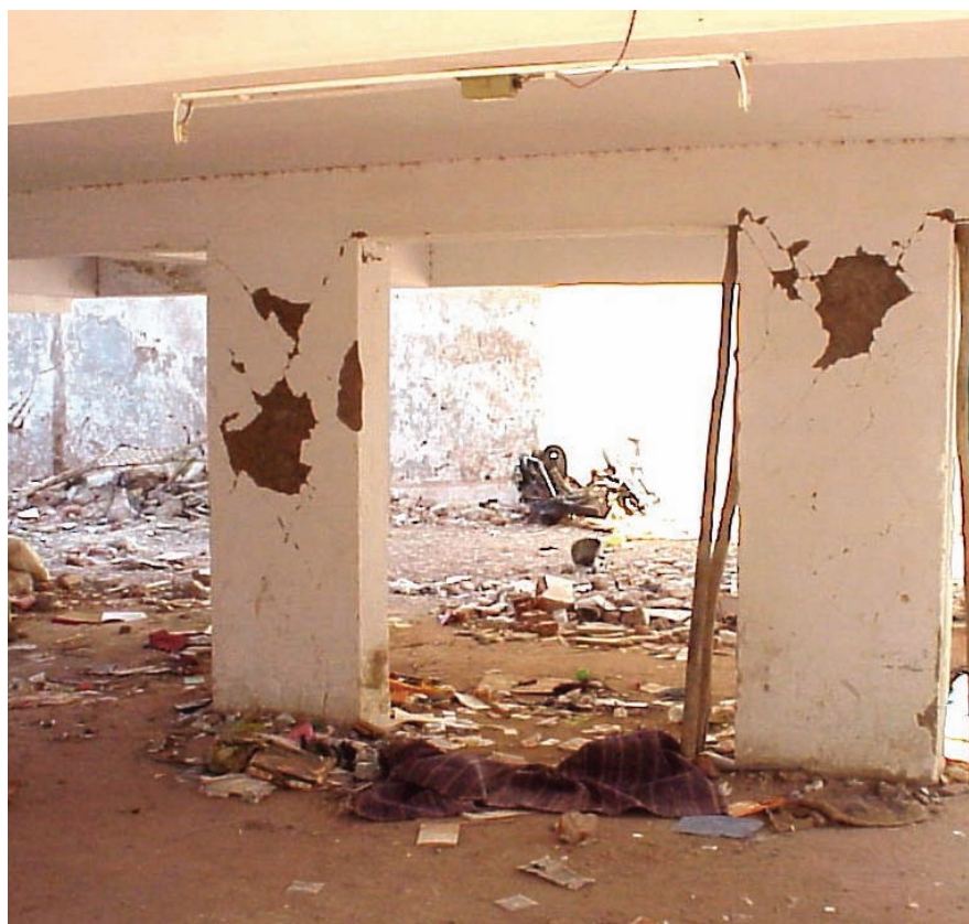
Fig. 8. Shear cracking of column. Courtesy: MAE Center.
