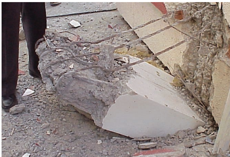
Fig. 7. Non-ductile detailing of column. Courtesy: MAE Center.
