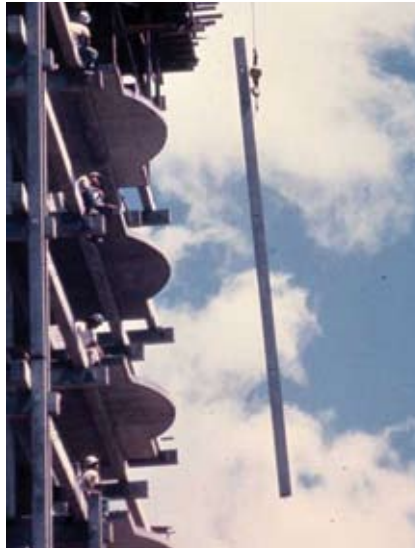
Fig. 1(a). Precast, prestressed trellis beam being erected on the Kahala Mandarin Oriental Hotel in Honolulu, Hawaii.
