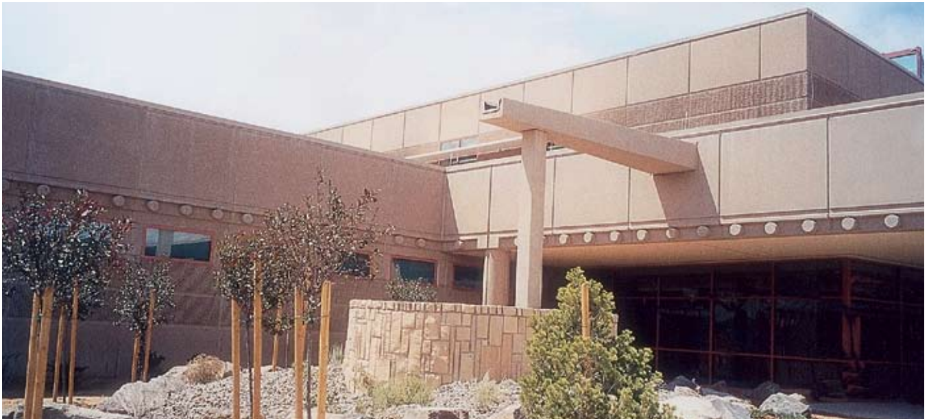
Fig. 18. Precast scuppers required a separate precast column for support because they were too heavy to cantilever from structure.
