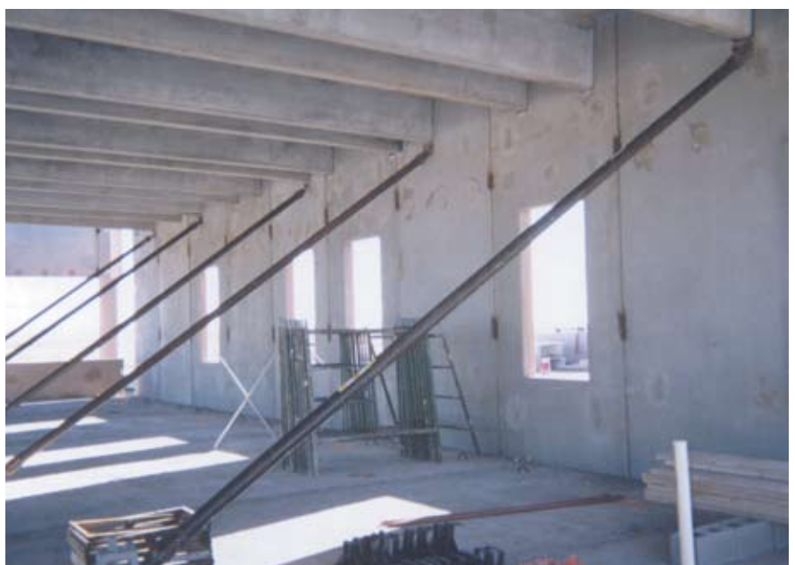
Fig. 11. Designers chose an all-precast concrete structural frame after looking at several steel options.
