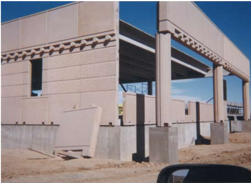
Fig. 16. Round precast concrete columns were used as exterior roof supports and also as interior supports, blending the two spaces.
