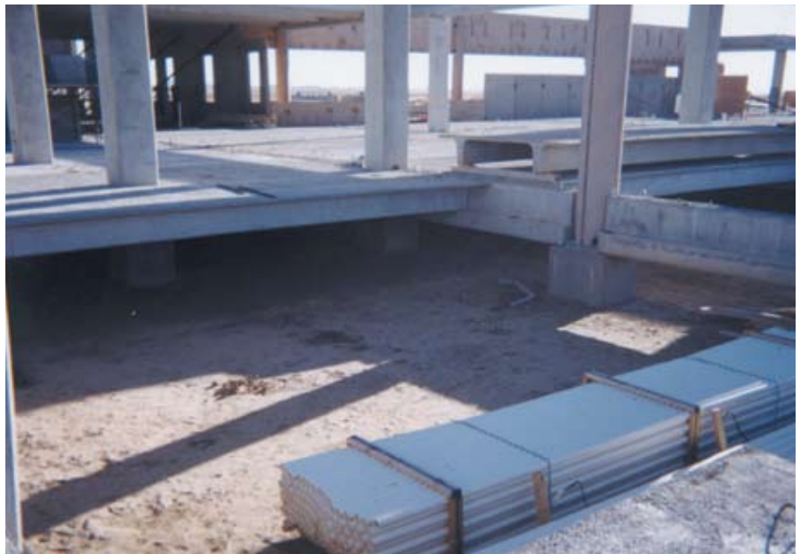
Fig. 14. A crawl space was created to provide mechanical access, and this space was aided by using double tees for flooring.
